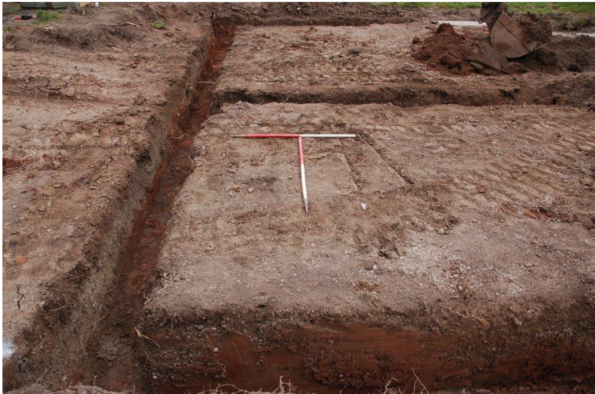
Plate 5. Strip foundation trenches at western end of site. View north. Scales 1m.
