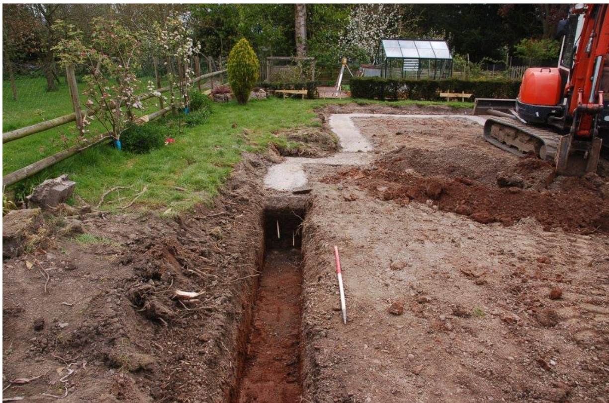
Plate 6. Strip foundation trench in the north of site. Trenching in the rear of shot has been concreted. View east. Scale 1m.
