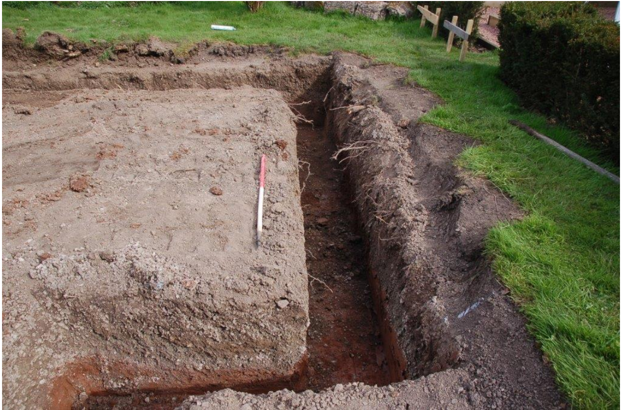
Plate 3. Strip foundation trench in the north-east of site. View north. Scale 1m.
