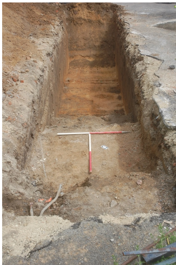
Plate 3: Overview of Trench 1, with live service in foreground and natural sand below post-medieval soil
