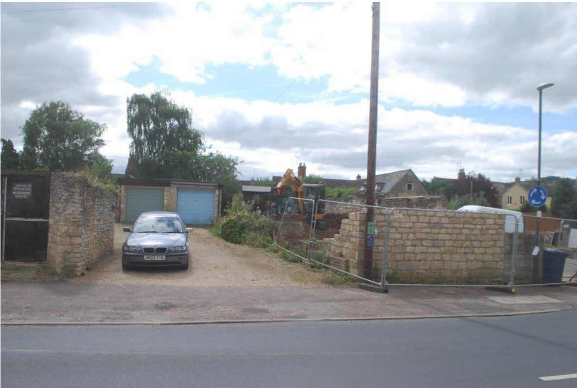
Plate 1 The site as works started, showing slope of ground, view south, no scales
