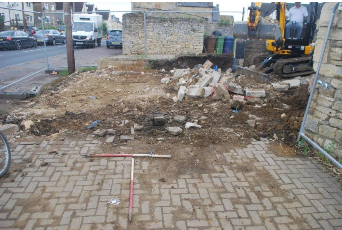
Plate 8: Ground reduction in area of former garage, view north-east, 2x 1m scales
