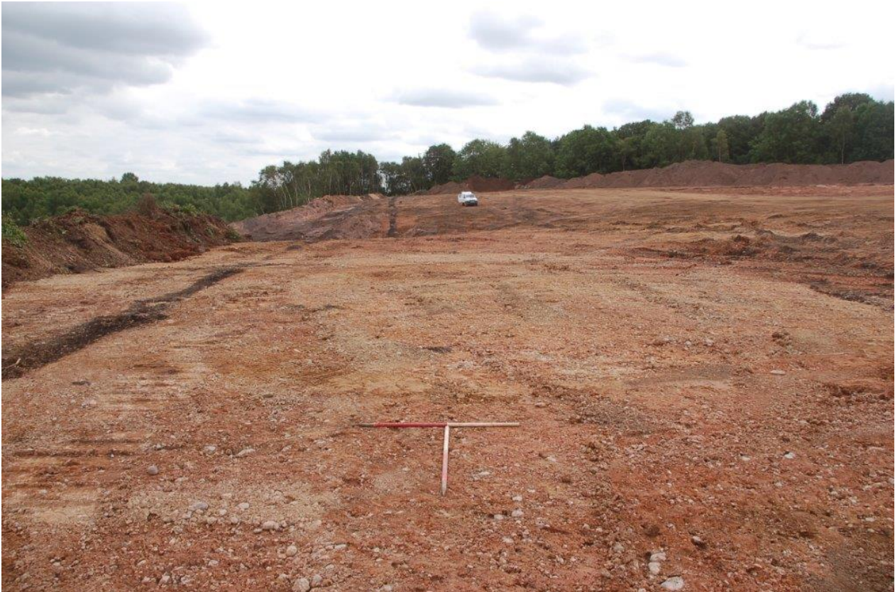
Plate 9. General shot of site strip, with ditch 119 visible to the north. View southeast. Scales 1m.
