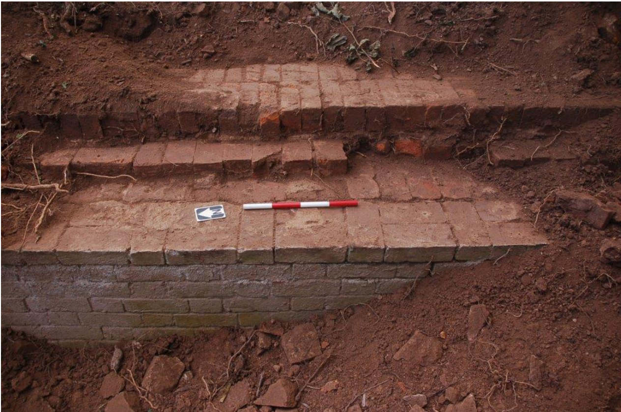
Plate 8. The original flanking wall (104), in the background, abutted by the later engineering brick re-facing (107) in the foreground, view south-east, scale 0.4m
