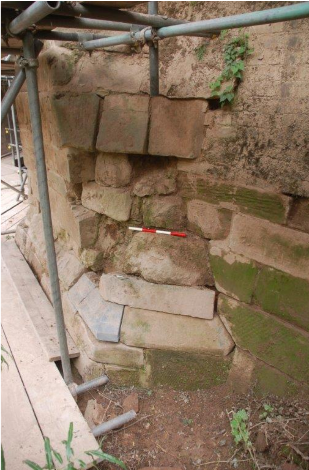
Plate 13. The heavily eroded masonry due to be replaced, at the foot of the south-west buttress, view north-east, scale 0.4m
