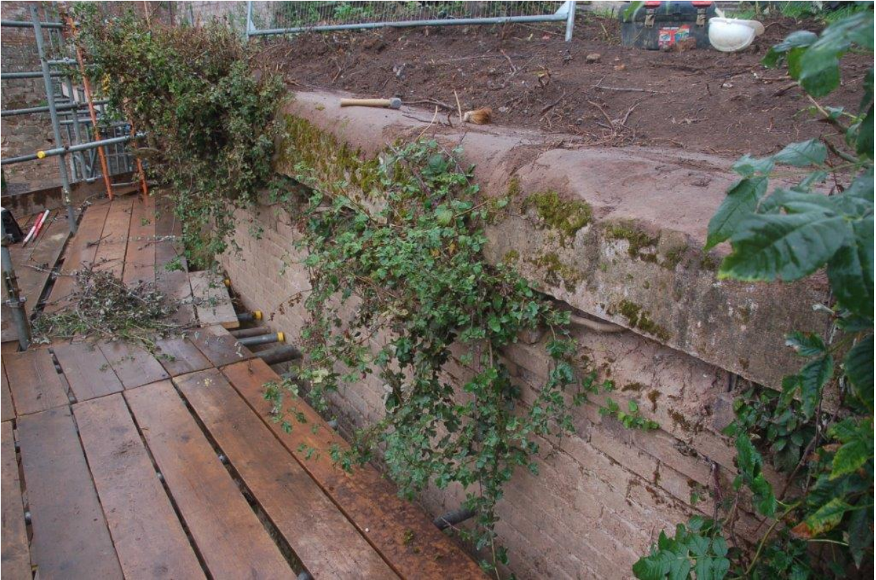
Plate 10. The damage caused to the flanking wall (107) and the coping stones (108), view north-east
