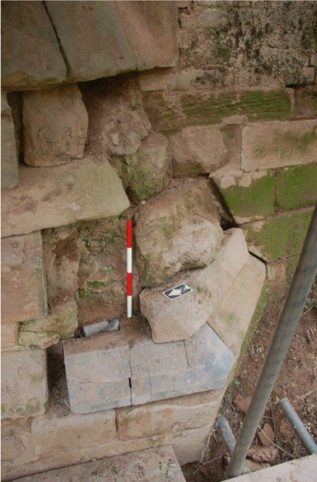
Plate 12. The heavily eroded masonry due to be replaced, at the foot of the south-west buttress, view south-east, scale 0.4m
