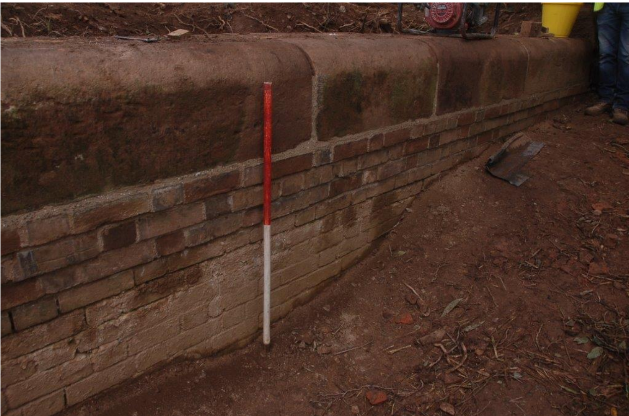
Plate 11. The repointed and repaired flanking wall (107) with reinstated coping stones (108), view south-south-east, scale 1m
