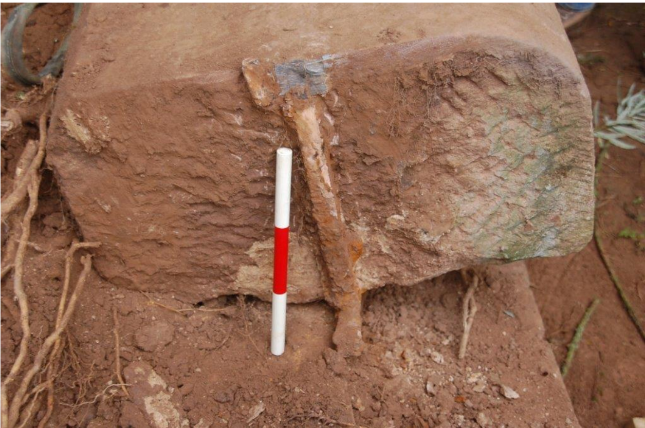
Plate 6. Iron bar within the joins of the coping stones, welded to both upper and lower iron strapping, scale 0.3m
