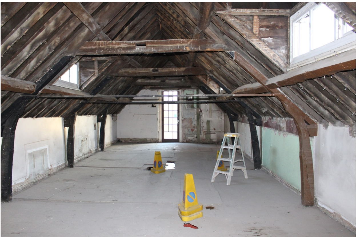
Plate 4: The interior of the northern half of the property, showing the third floor of 3, Foregate Street
