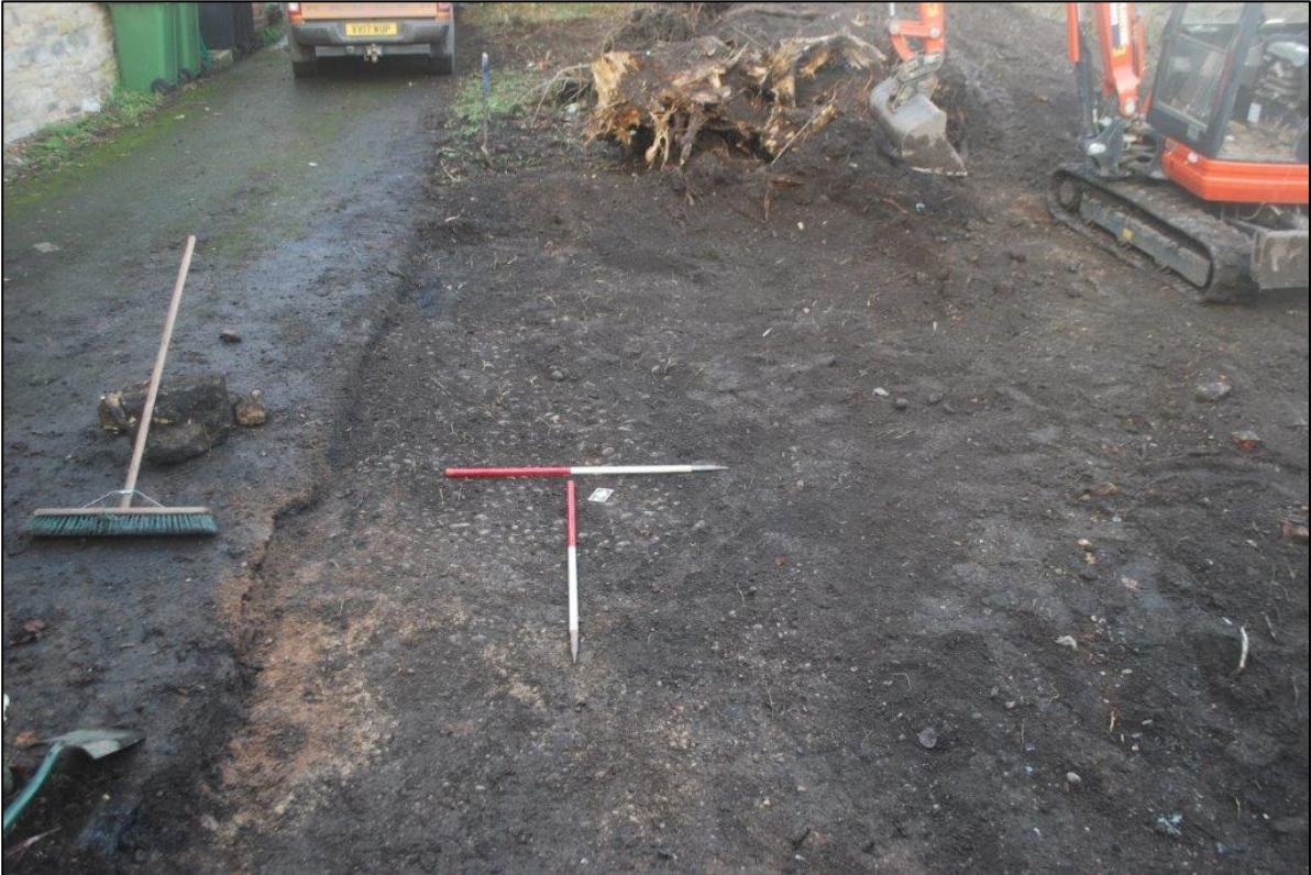
Plate 5 Area of cobbled surface (104) after cleaning up, view north-west, 2x 1m scales
