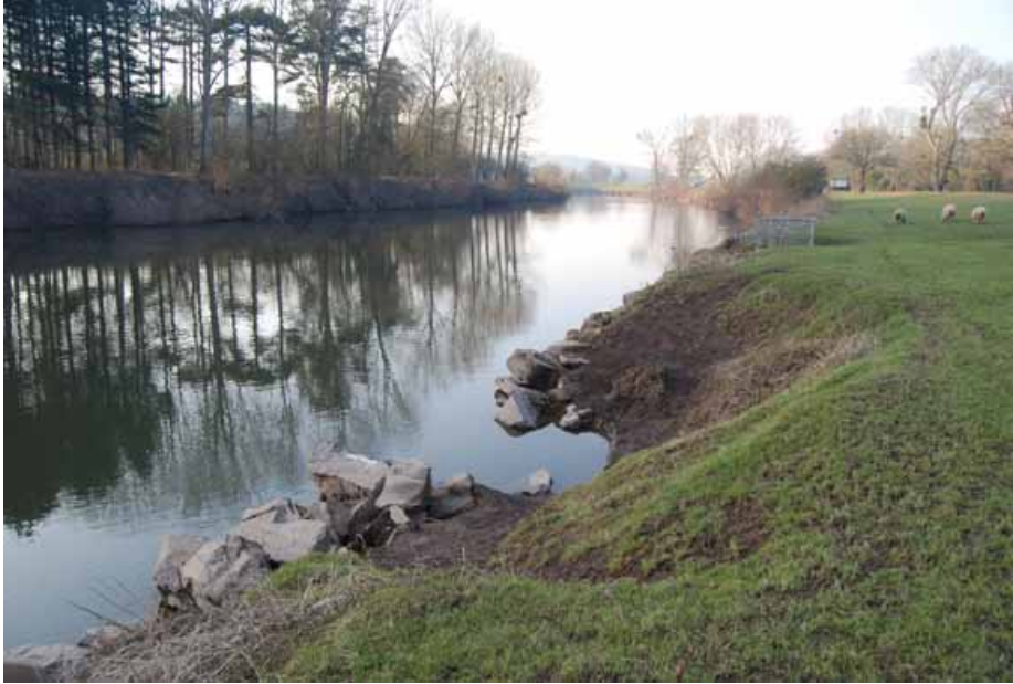
Figure 18 Stone revetment at base of the river-bank typical of both banks of the river in this part of the Severn
