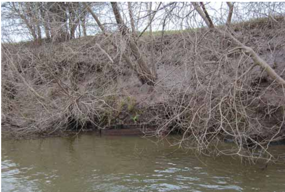
Figure 16 Exposed brickwork under bank at Mythe Hook (UID 283; east bank). This brick structure 5-6 courses high and about 5m wide was visible at the bottom of the bank. It had been cut into the bank and projected about 1m into the river. Now obviously truncated it was covered with collapsed bank material. Though unclear what this structure represents, it was obviously not recent, and presumably relates to the brick and lime kilns shown on Young's map of 1784. An adjacent clay pit is depicted on the first edition OS map of the 1880s, and is now a long pond. It may have been the pier of a jetty, in which case other foundations might survive in the river-bed
