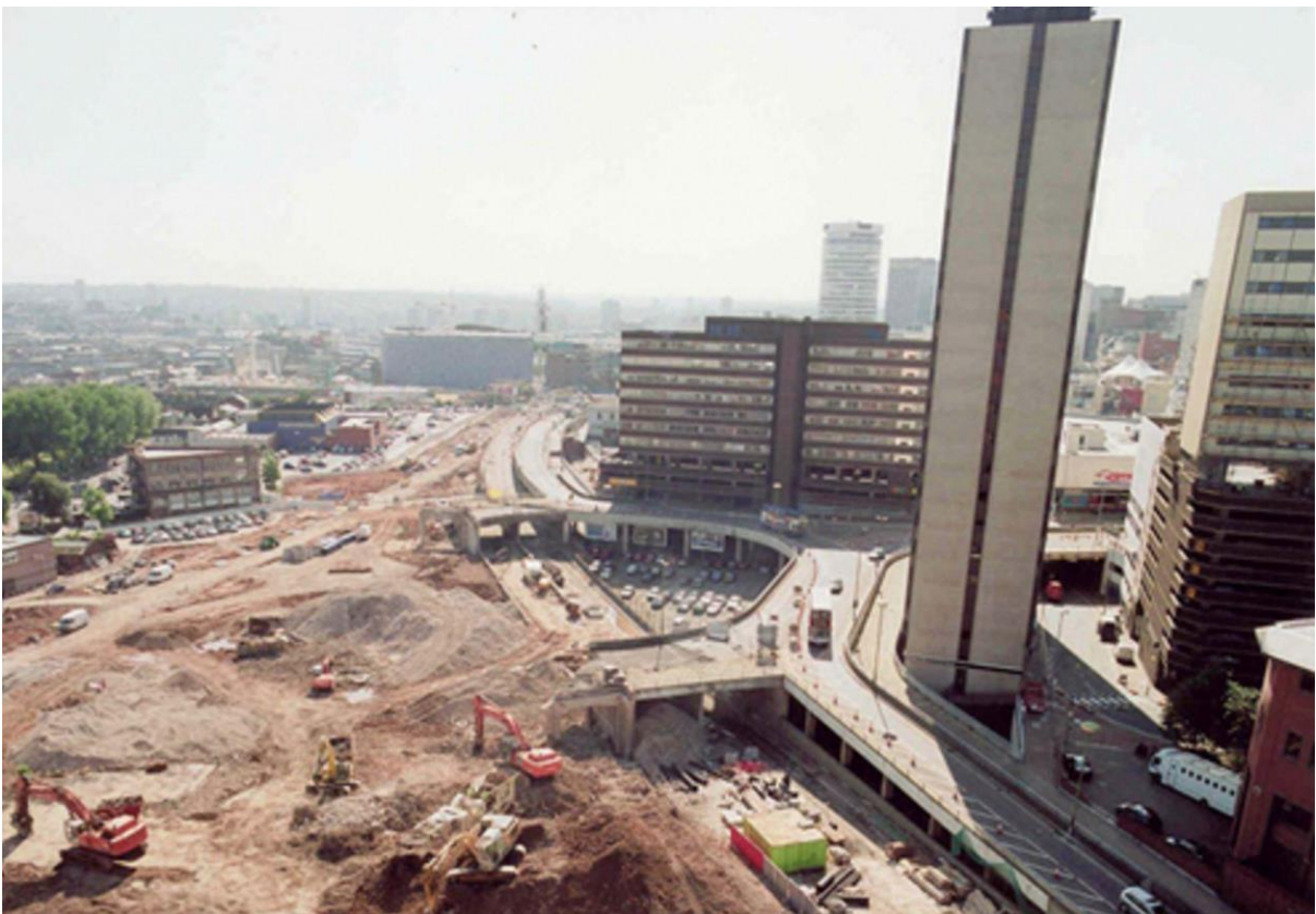
Plate 18: demolition of the elevated road (Masshouse Circus) crossing the site in 2002, facing south.
