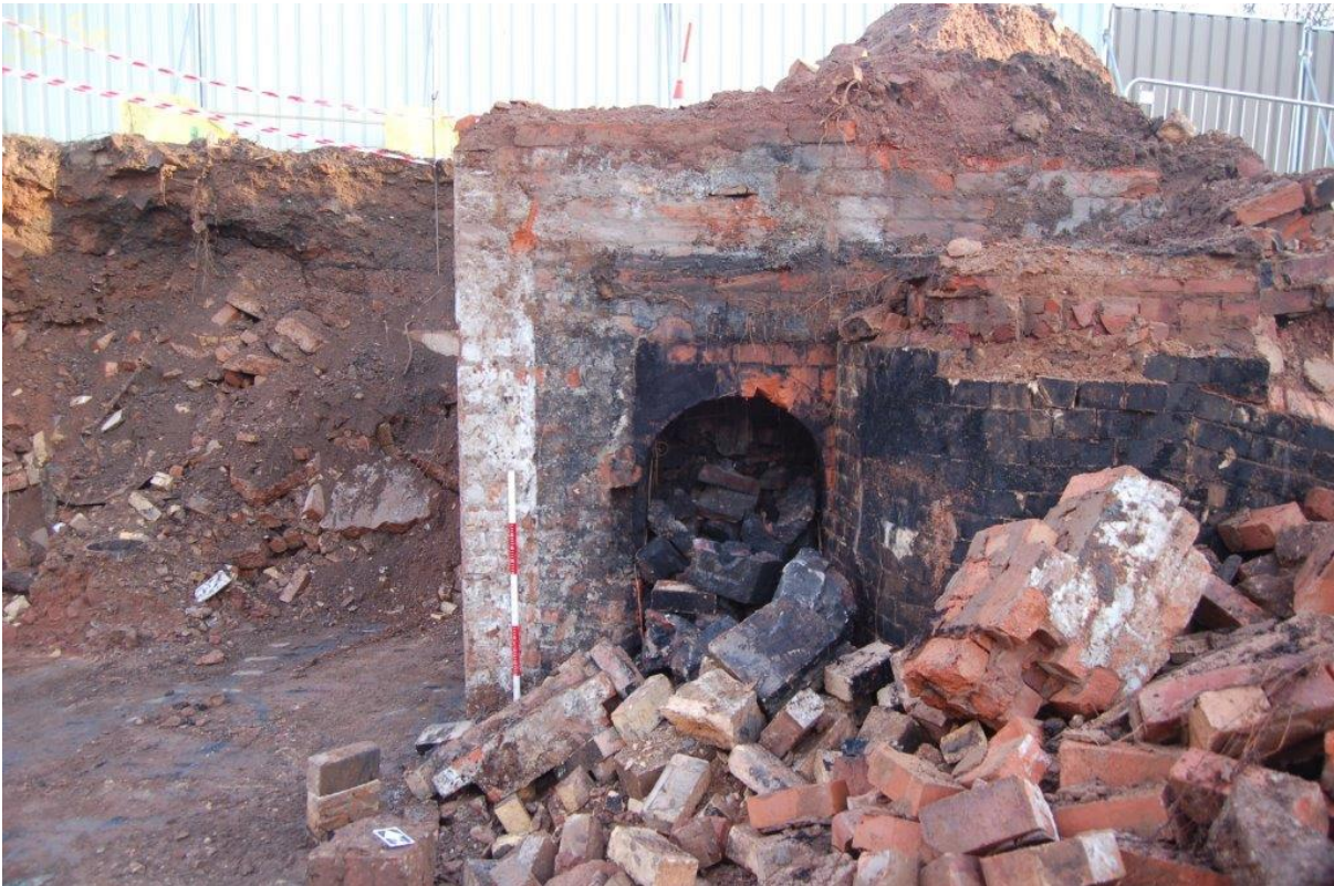
Plate 17: vaulted archway beneath chimney base. Taken after the demolition of part of the structure, 1m scale, facing north east.
