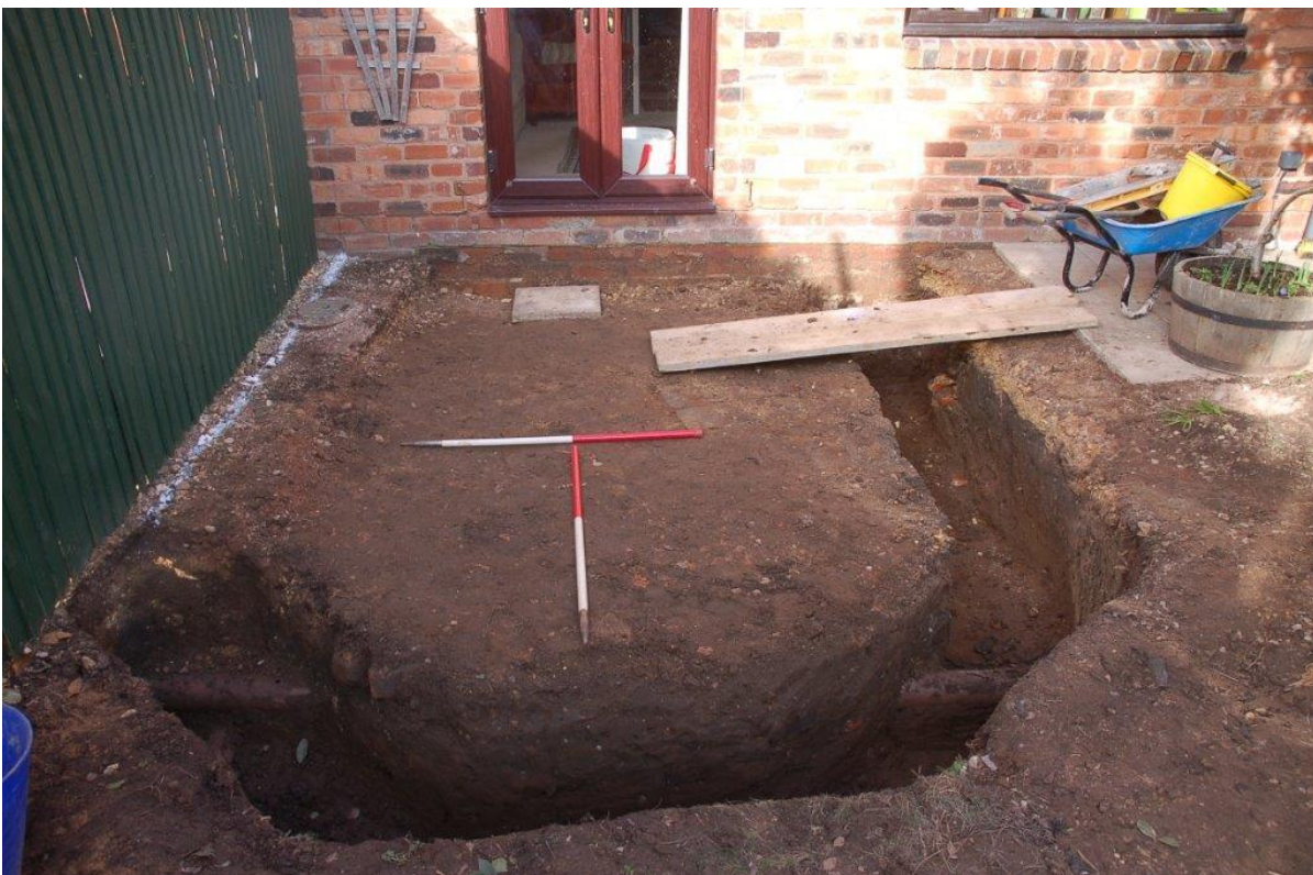
Plate 4 The footing trenches excavated. Western side was left due to presence of modern drain. 2x1m scales, looking north.
