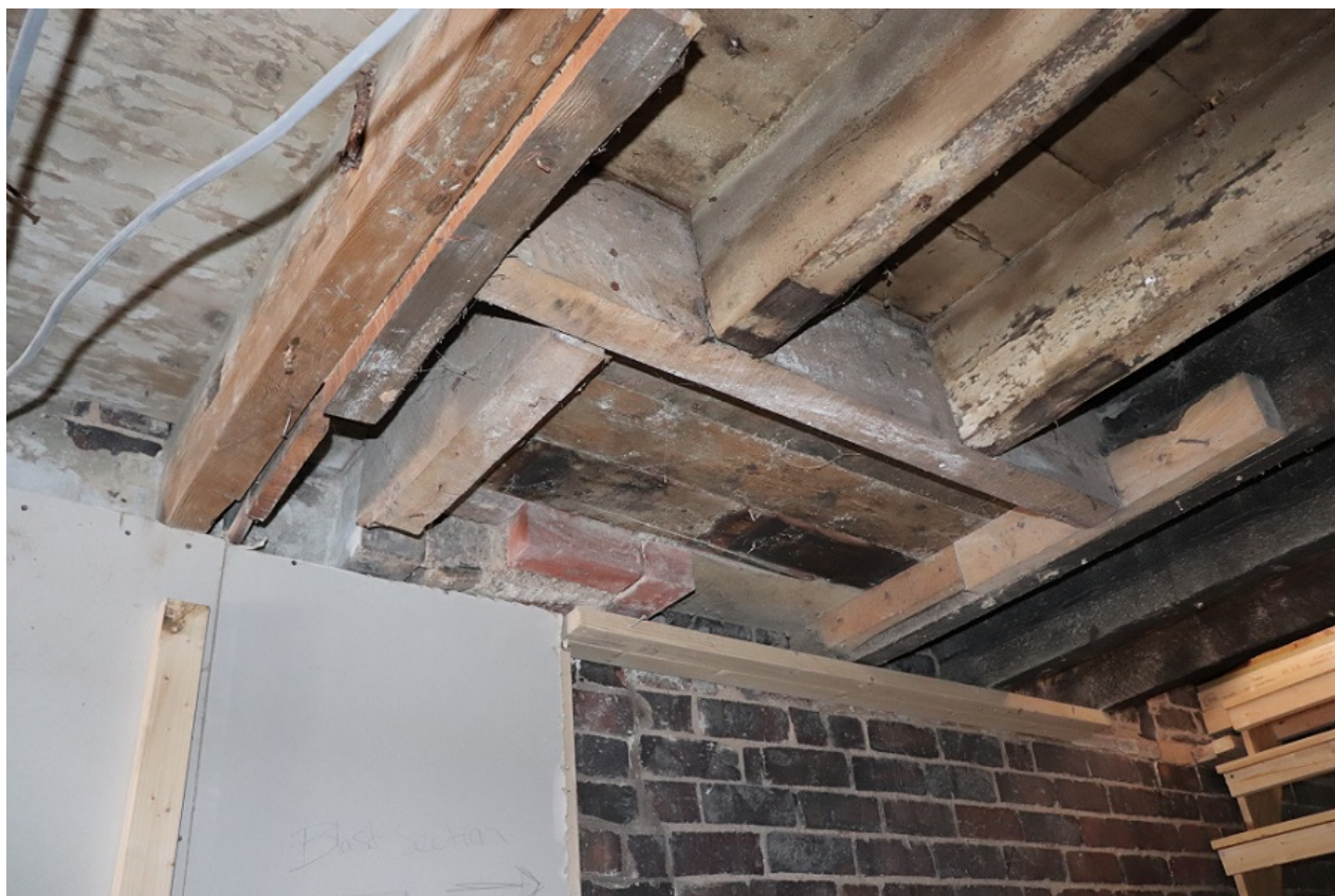
Plate 8 Ground floor interior, detail of ceiling joists below fireplace on first floor above, no scale
