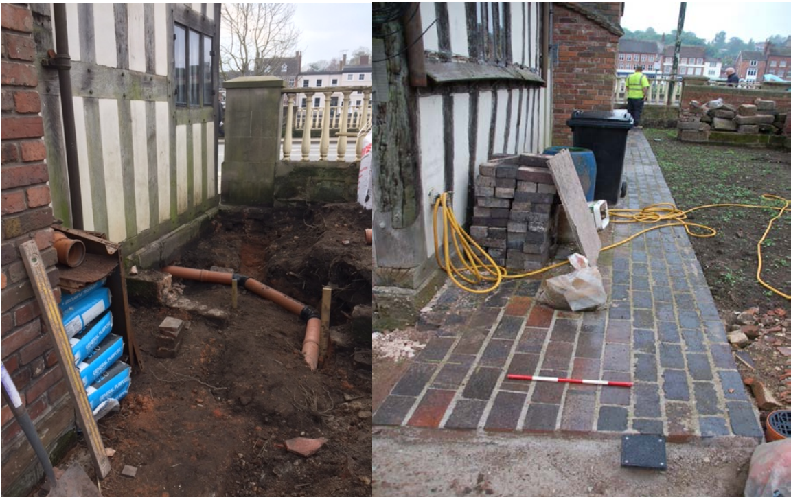
Plate 2: North-western side of the property during groundworks (left) and as seen during the archaeological watching brief (right). Facing south-west.
