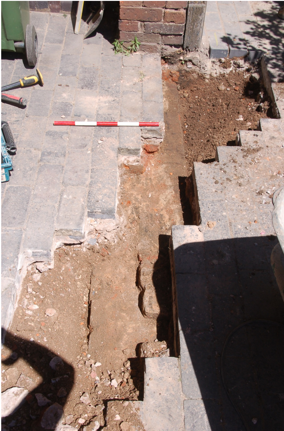
Plate 5: Brick wall (3) on the south-east corner of the property, 0.5m scale, facing north-east.
