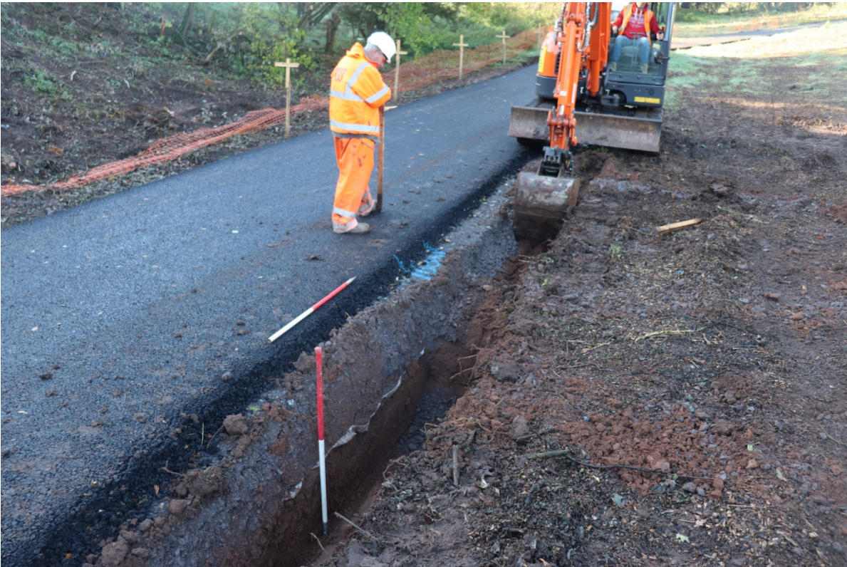
Plate 5 The drainage trench during excavation adjacent to new road, view north, 2x 1m scales
