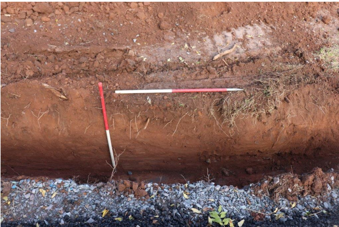
Plate 8 Sample section of drainage trench in the north of the site, view south-east, 2x 1m scales
