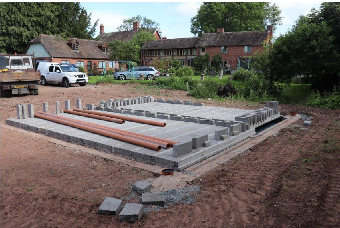
Plate 2 Existing garage foundations in east of site, looking north-west towards the Old Tannery
