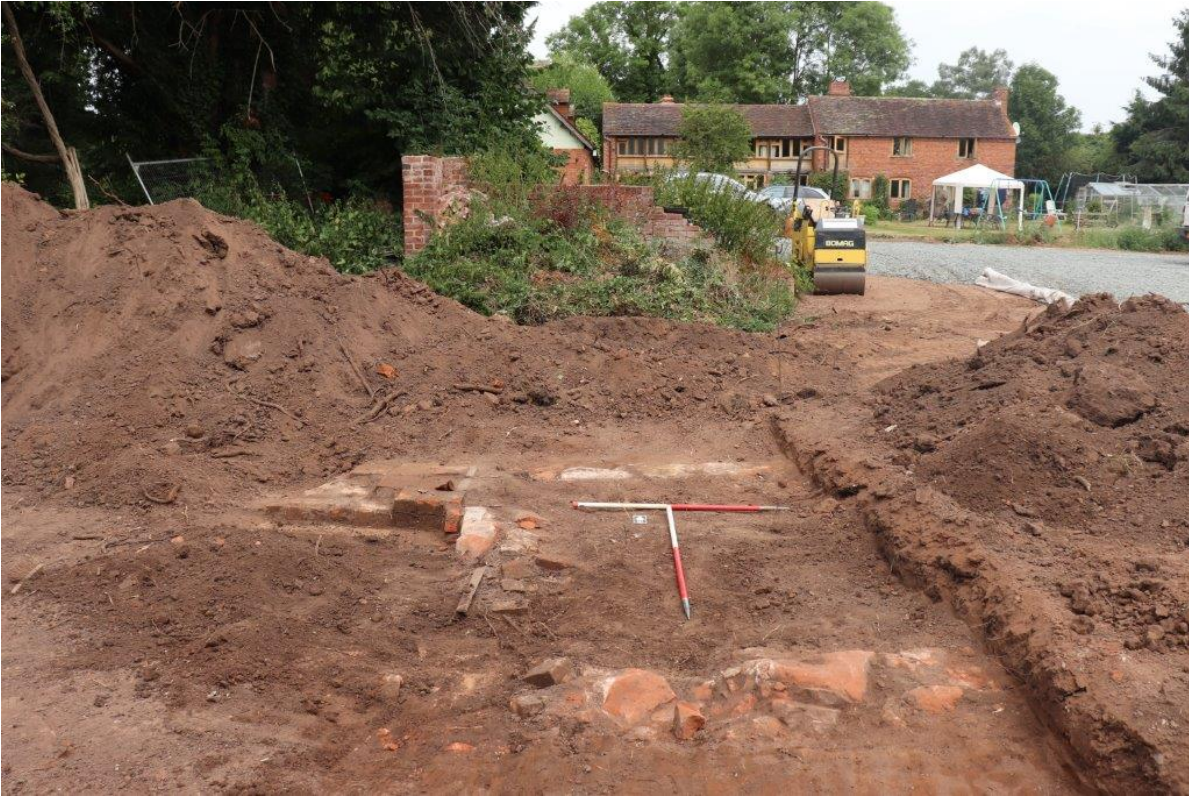
Plate 9 Building footings 207-209, looking north towards modern brick built shed and the Old Tannery building, 2x 1m scales
