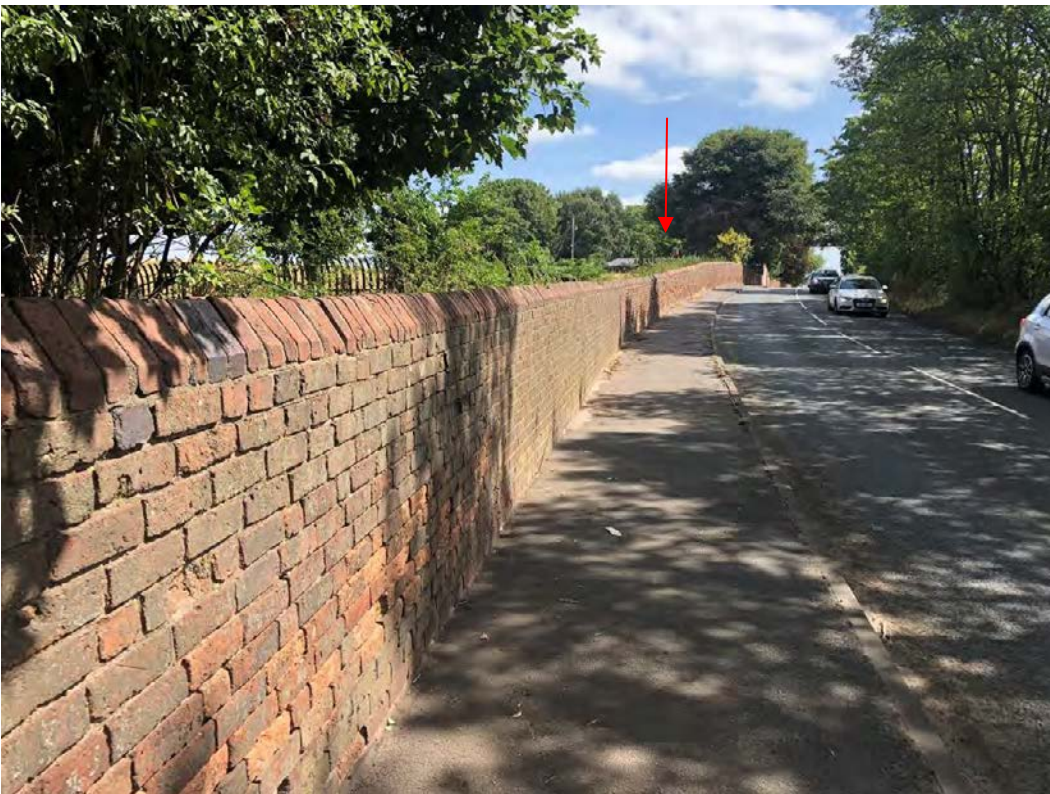
Plate 10: The brick wall around the former park still largely survives intact. Broom Cottage also survives as a private residence, hidden behind the park wall
