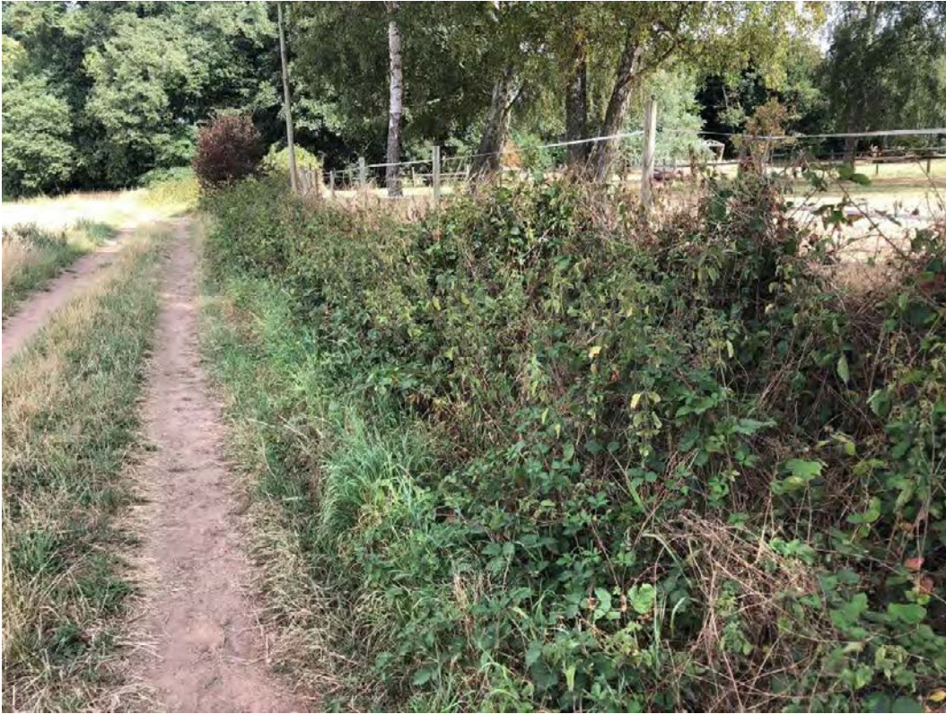
Plate 13: The remains of a ha-ha are just visible surviving below undergrowth on the northern boundary of the site
