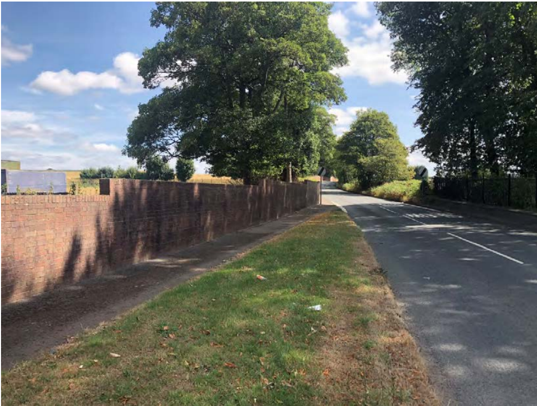
Plate 11: Parts of the park boundary wall have been unsympathetically rebuilt
