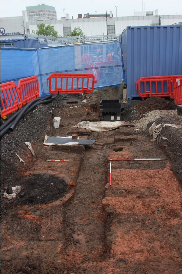
Plate 1: General view of the site area during the watching brief, facing north, with the cut for the cable ducting trench visible running through the middle
