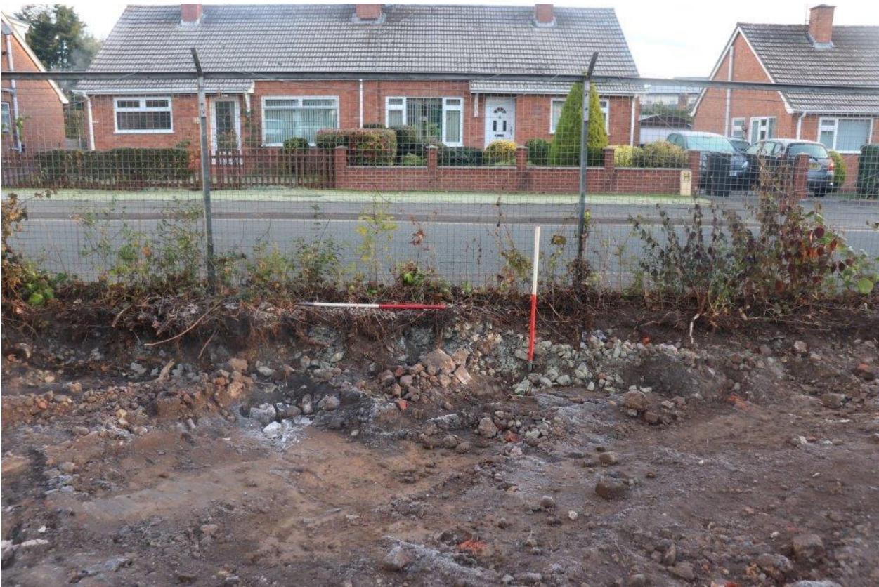
Plate 5 Southwest facing section of groundworks adjacent to Himbleton Road. In area for car parking with 2 x 1m scales.
