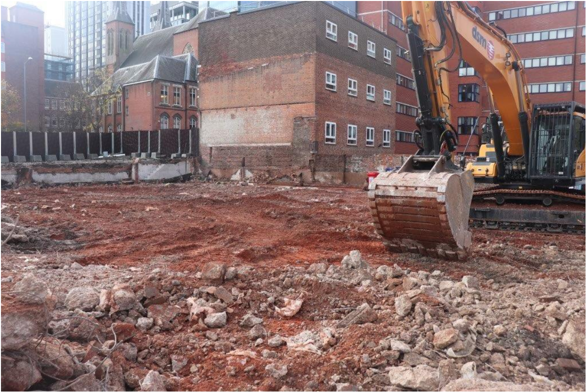
Plate 1: Western end of site following warehouse demolition and hardstanding removal. View southwest
