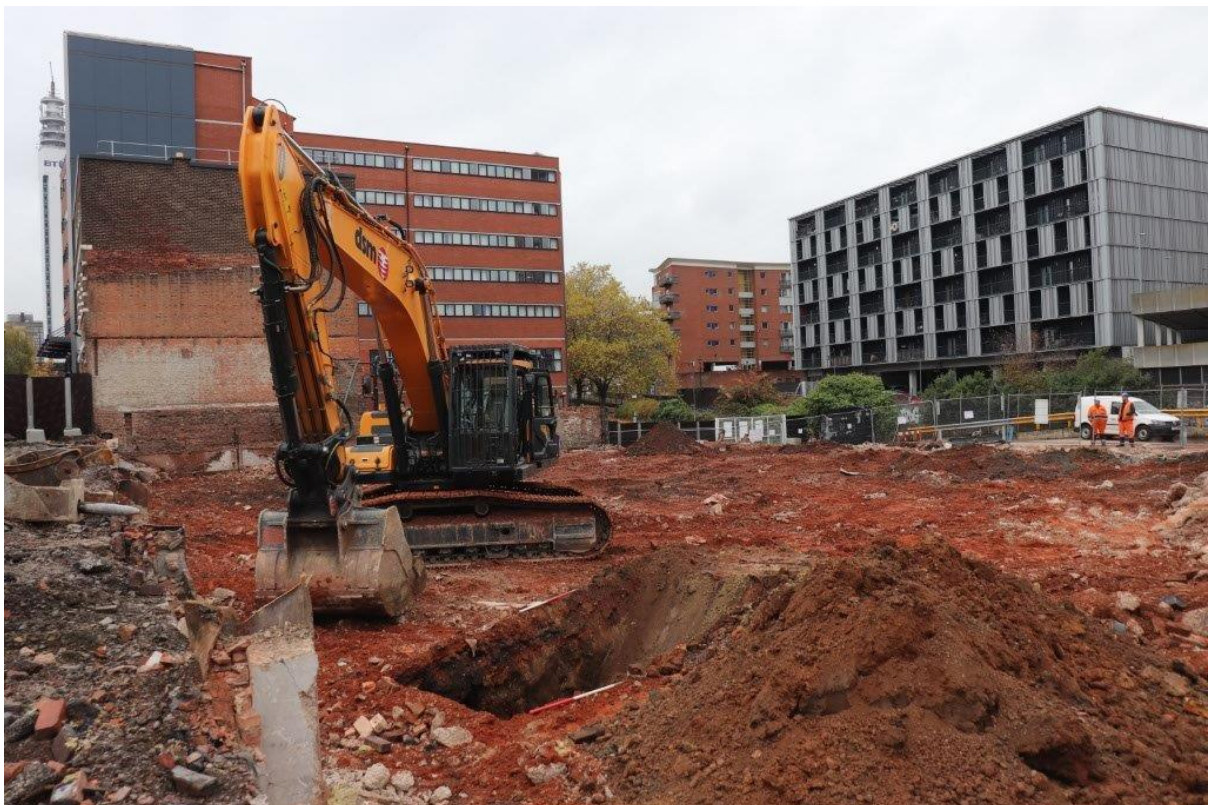
Plate 8: Location shot of Trial Hole 5 looking northwest towards Birmingham and Fazeley canal
