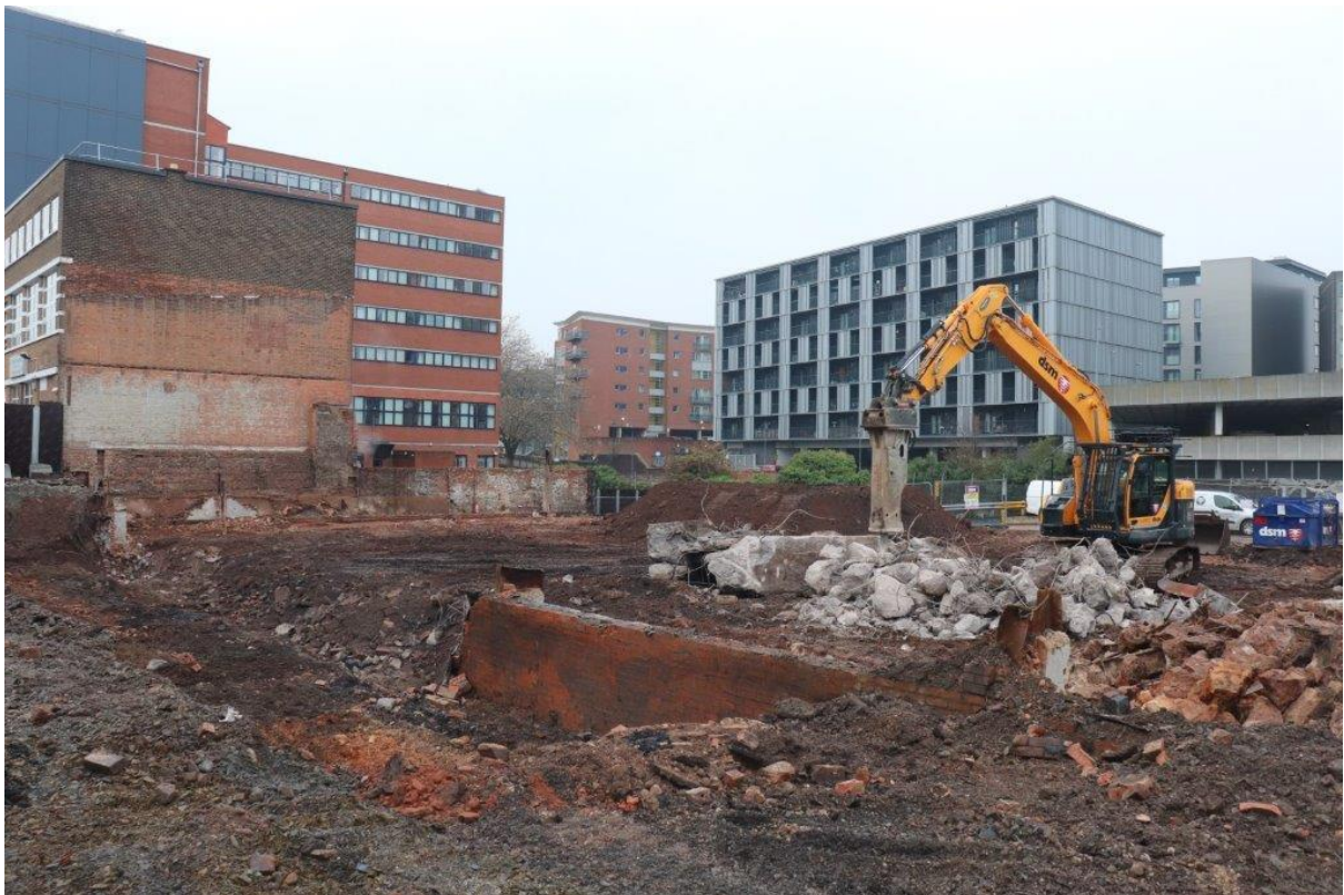
Plate 10: General shot showing existing concrete retaining wall in being removed. View northwest towards canal-side
