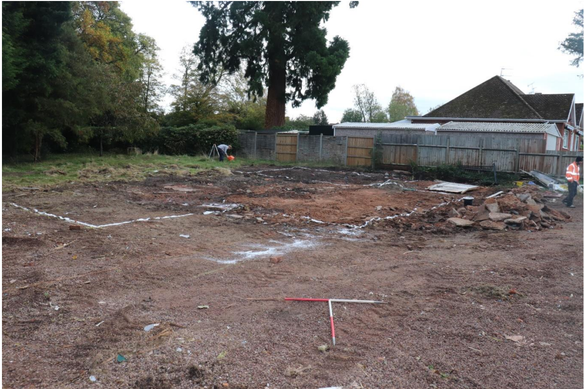
Plate 1: General view of site after demolition but prior to footing excavations. Looking northeast, 2 x1m scales
