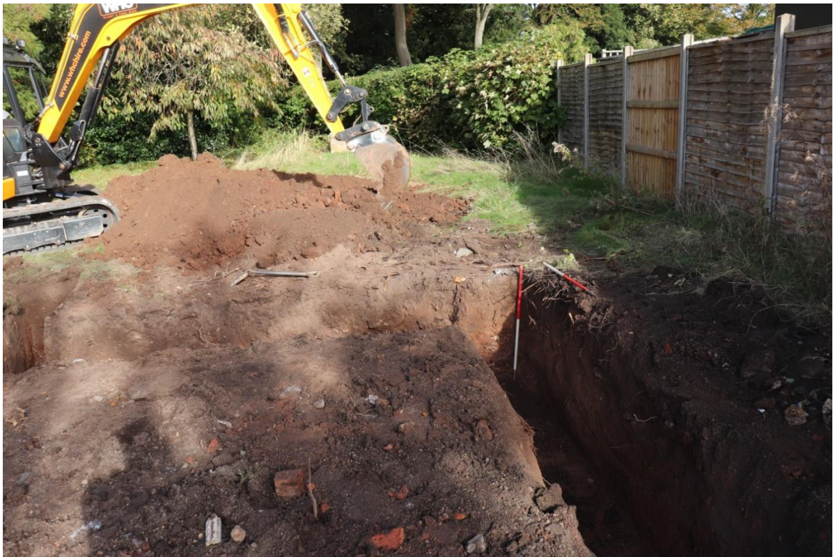
Plate 4: View of northern foundation trench after excavation. 2 x 1m scales looking north
