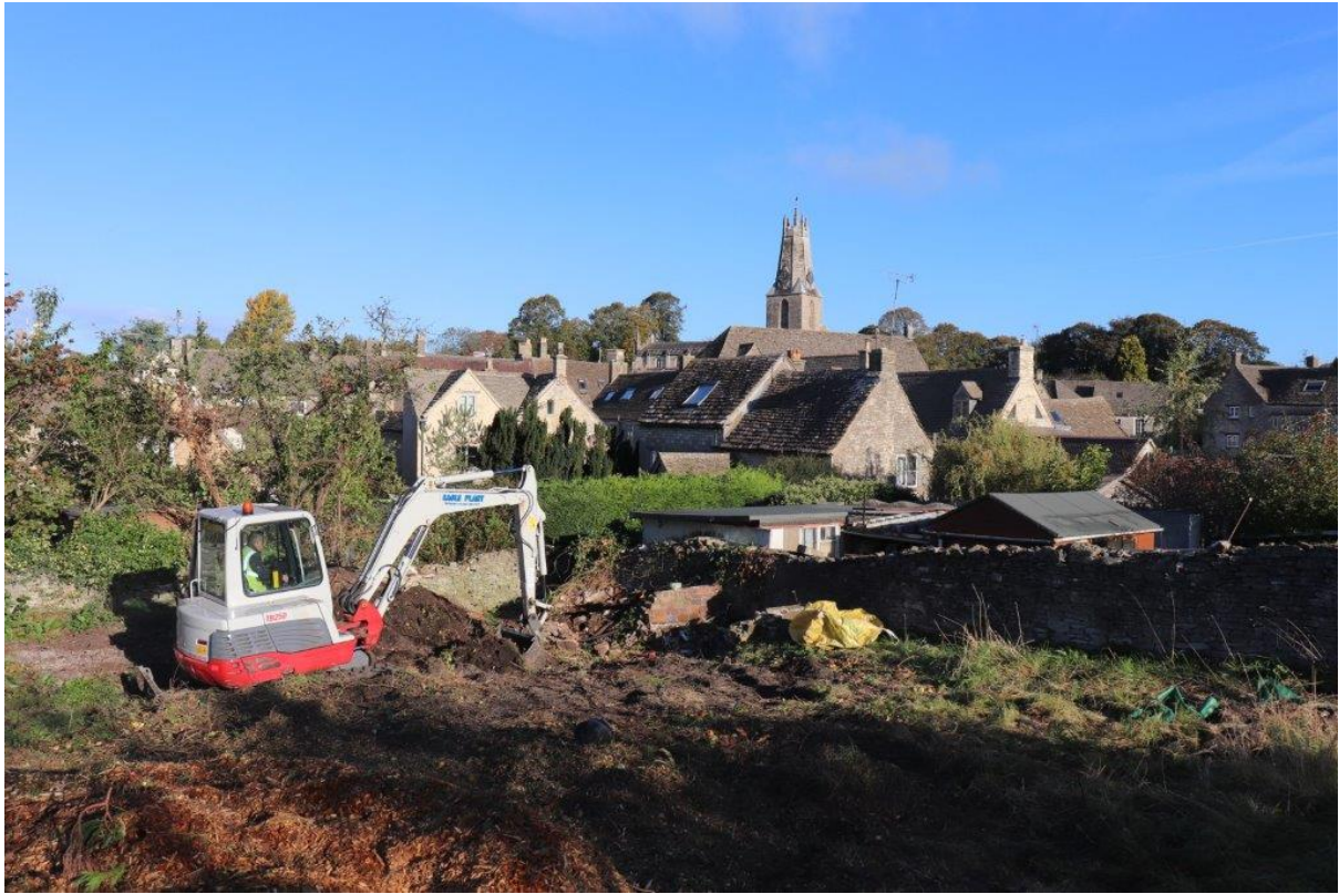
Plate 1: The garden area prior to reduced groundwork excavations. Looking northwest towards church
