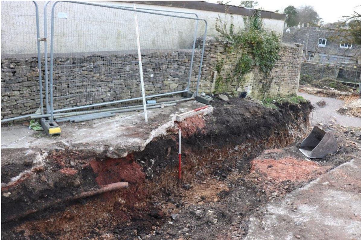
Plate 13: Service trench showing 20 th Century made ground deposit looking southwest, with 2x1m scales
