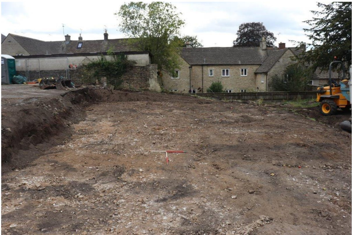
Plate 6: Maximum ground reduction area looking south, showing evaluation Trench 1 in foreground and Trench 2 to west of 1m scales
