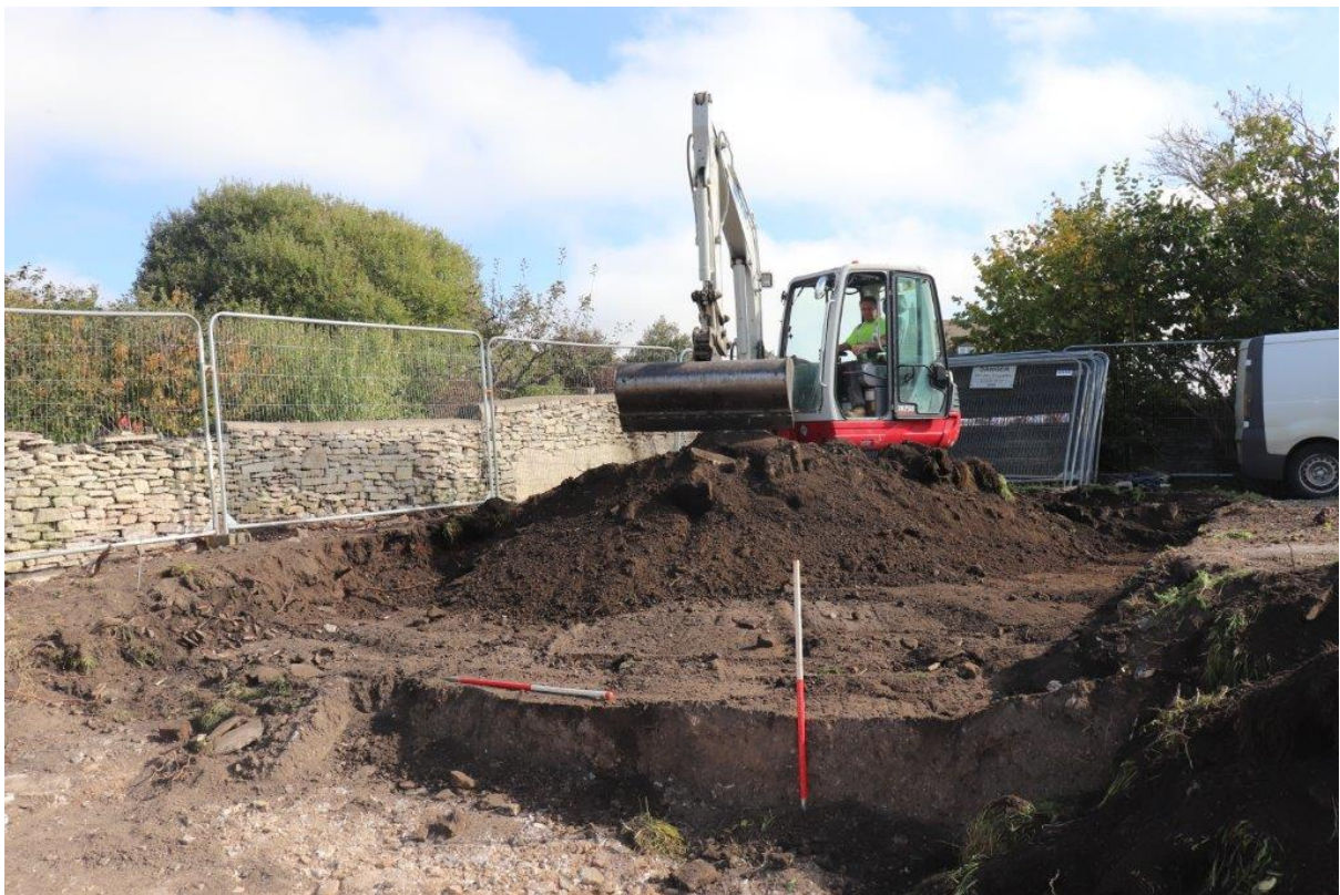
Plate 10: Area of car park showing removal of topsoil and made ground to maximum depth. 1m scales looking northeast
