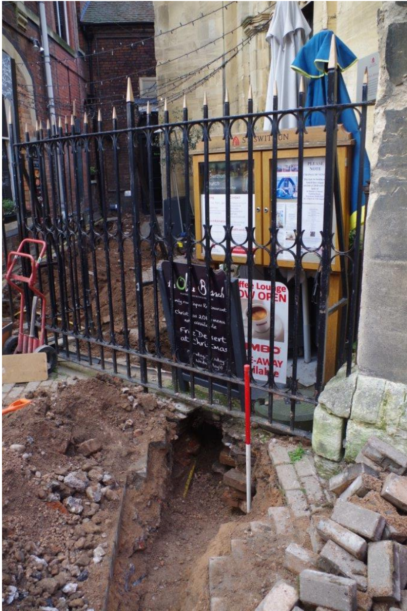
Plate 4: View north of trench, including boundary wall 113, seen from Church Street; 1m scale
