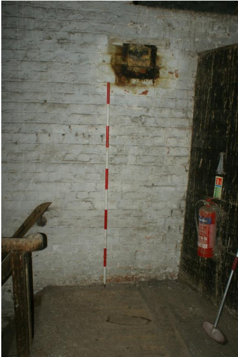
Plate 33 Building B fifth floor possible drive shaft hole, looking west
