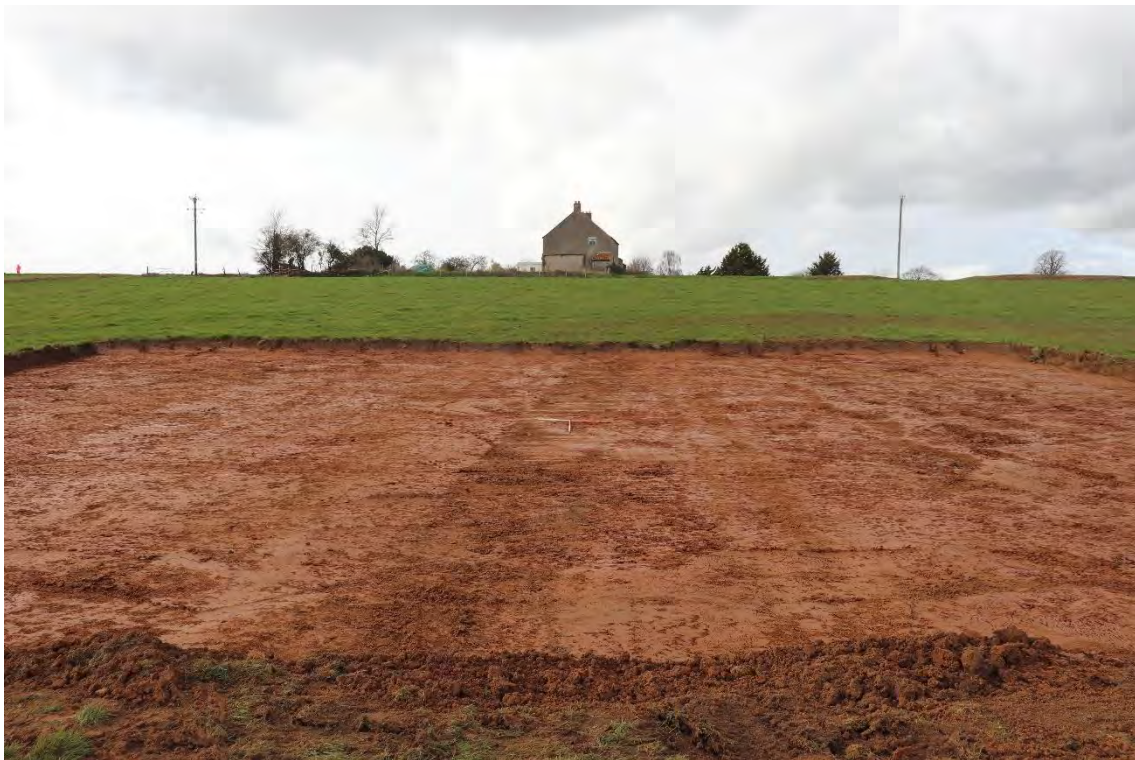
Plate 28: Trench 2, looking west towards Harry Stoke. Note the natural topography sloping upwards away from the camera. The evaluation trench excavated in 1996 is visible cutting the natural mudstone.
