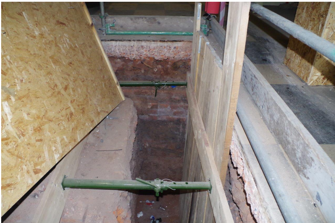
Plate 18: Trial Hole 6 showing wall in section, with garden soils and natural ground beneath, looking east
