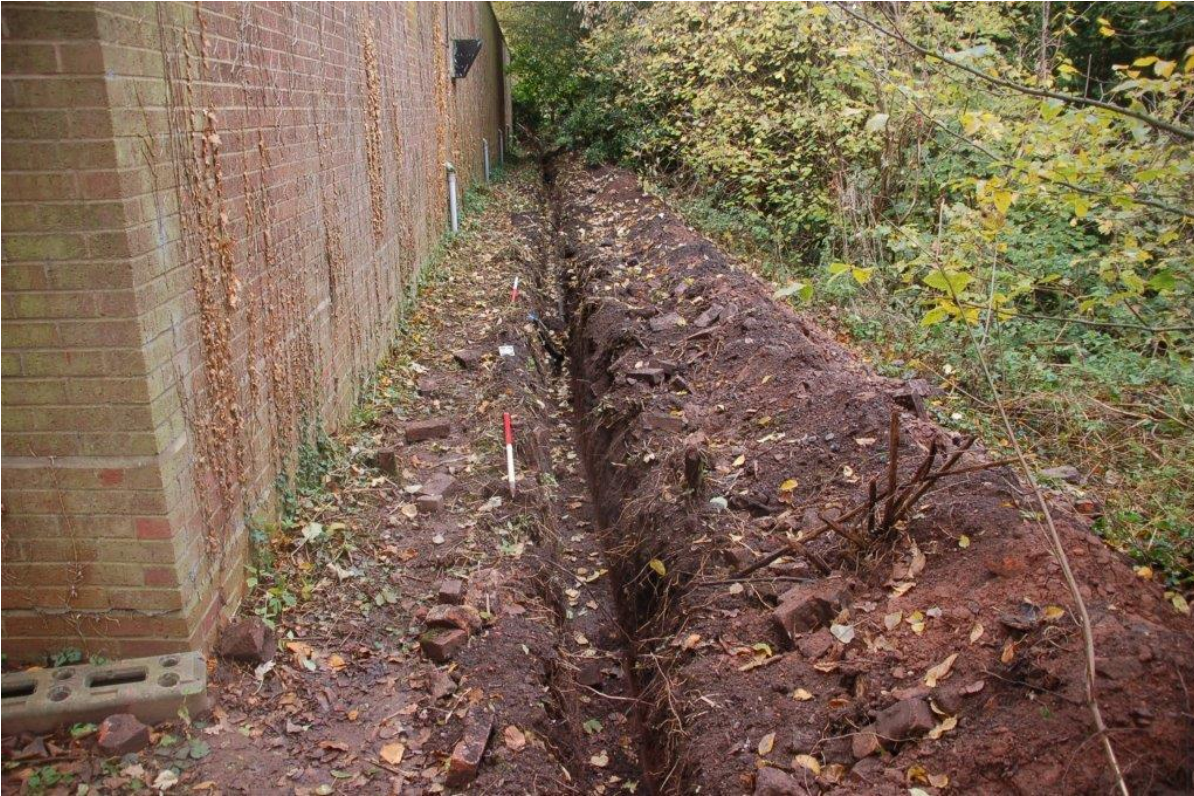
Plate 1 Trench 4 through proposed gas tank location. 2 x1m scales looking west. Gas tank location is at 1m scale in the foreground.
