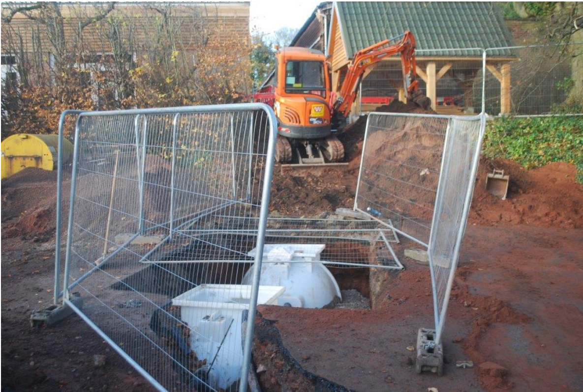
Plate 5 Sewer service trench in carpark with modern hardcore, surfacing and natural sands.
