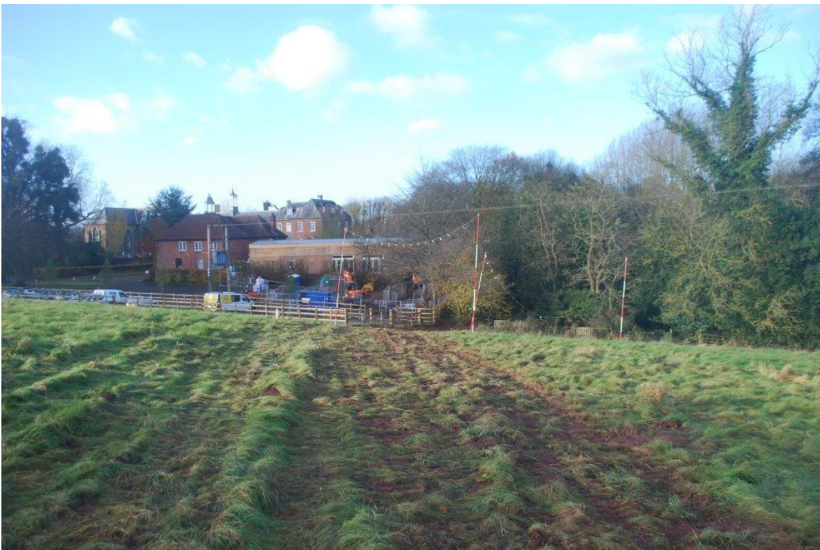
Plate 6 Location of service trench after backfilling. Ran across open field to existing sewer. View Southeast towards Hartlebury Castle.
