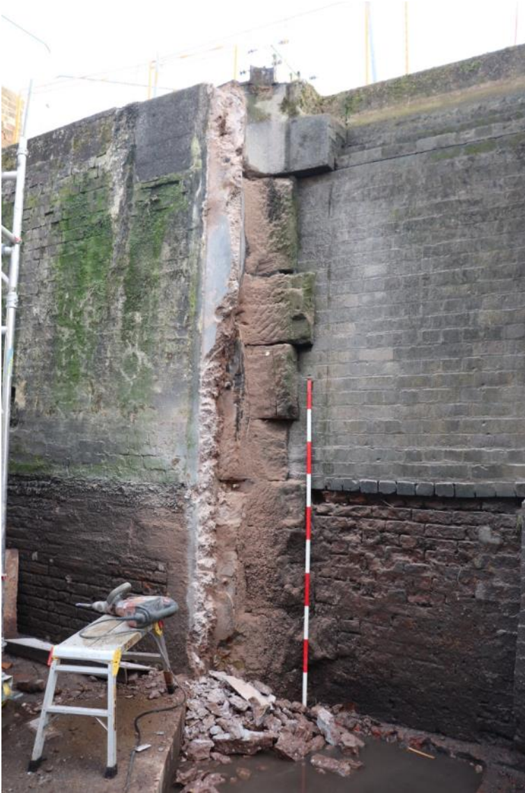
Plate 7 Stonework at the pivot of the tail gates, looking north-east, 2m scale
