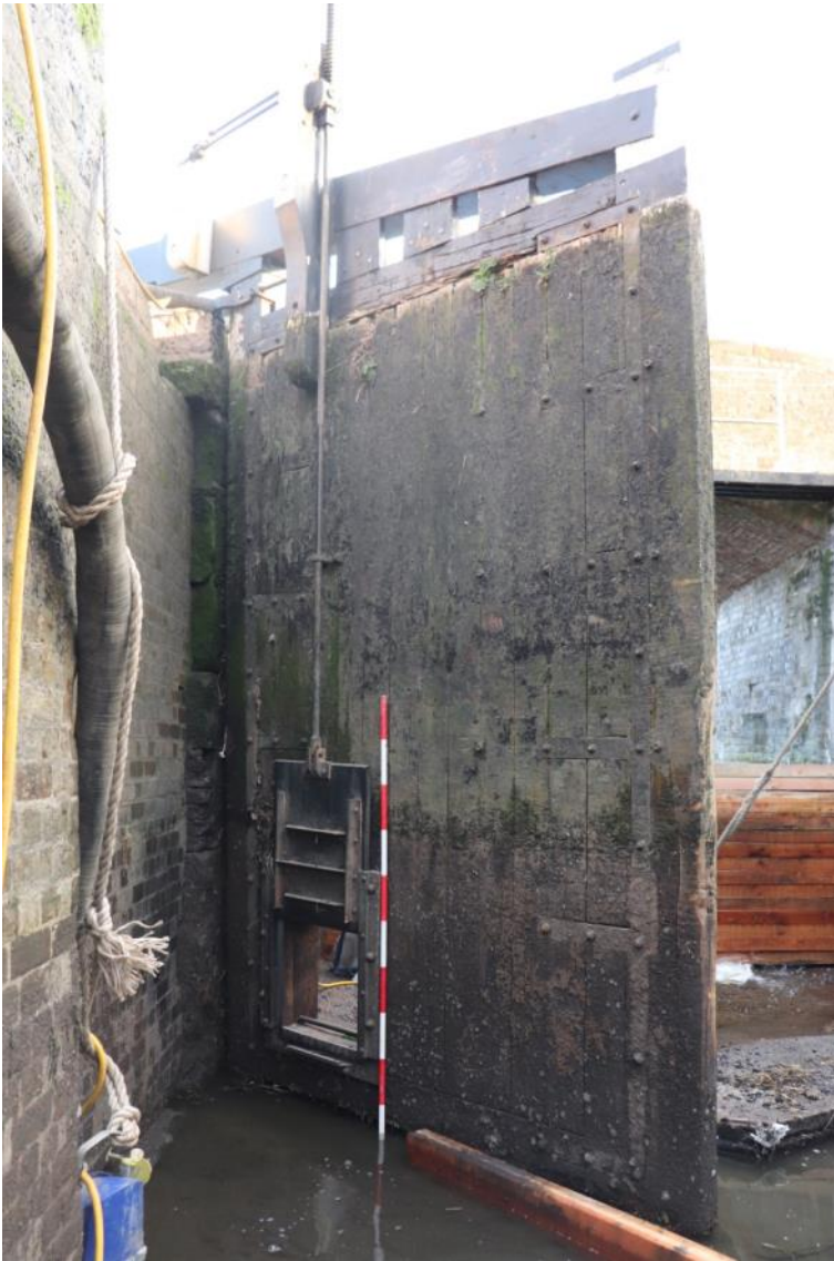
Plate 9 Tail gate with single paddle, looking north-east, 2m scale
