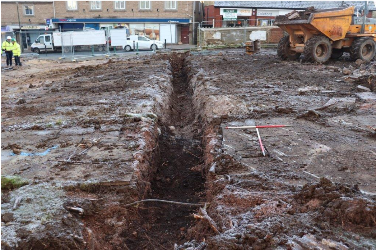
Plate 3: Trench 1 electricity cable, aligned east to west across site; view east; 2x 1m scales
