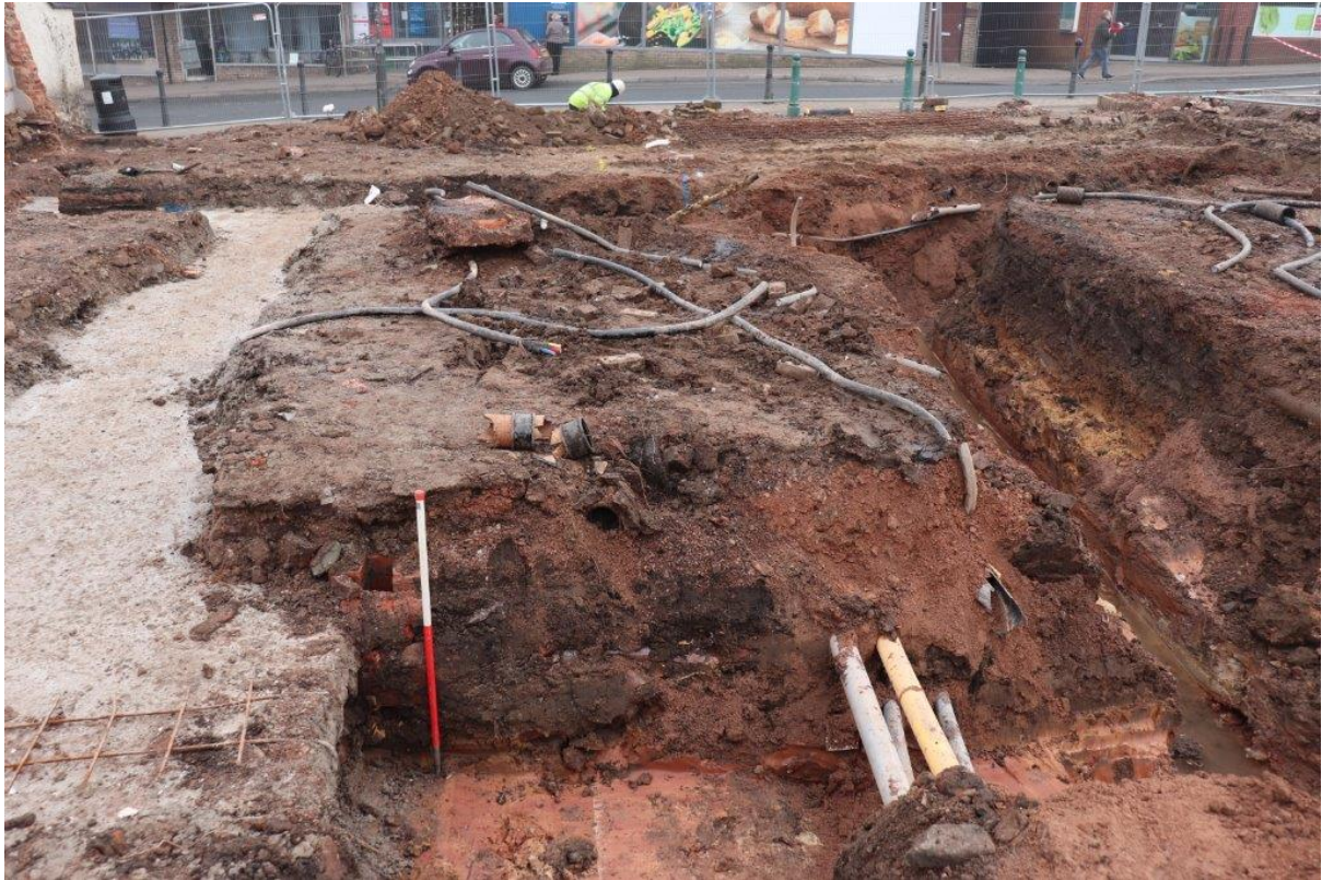
Plate 11: Trench 2 modern service trench, drainage and sewer truncations; view east; 1m scale
