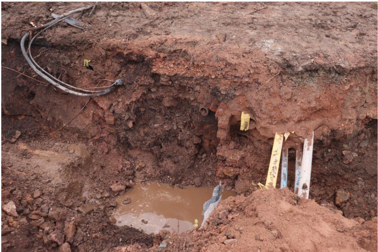
Plate 10: Trench 3, brick water storage drainage chamber structure (312); cut by modern sewer; view west; no scales
