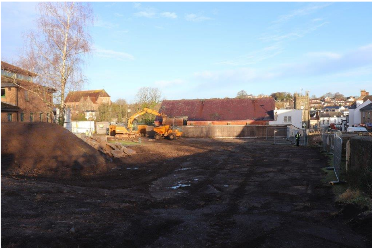
Plate 2: View north of site prior to excavations; machine removing hardstanding in background; no scales
