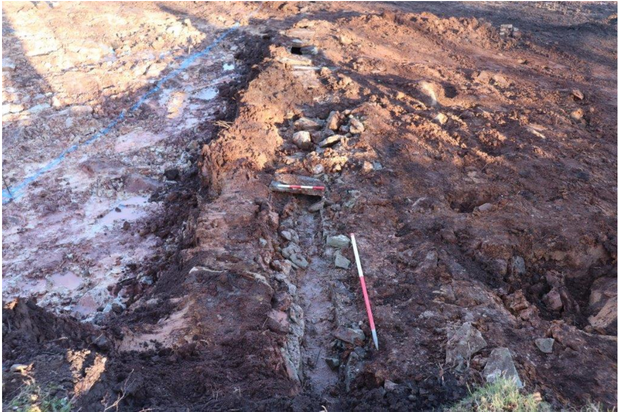
Plate 7: Trench2 stone culvert (205) relating to original Lawnstone building; view north; 0.4m and 1m scales
