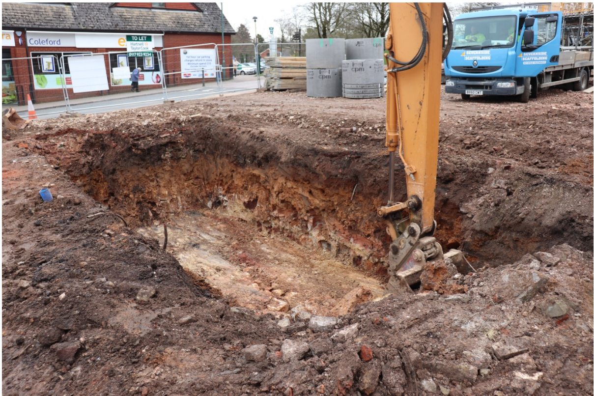
Plate 12: Attenuation tank excavated showing made ground and natural deposits; view south-west; no scales
