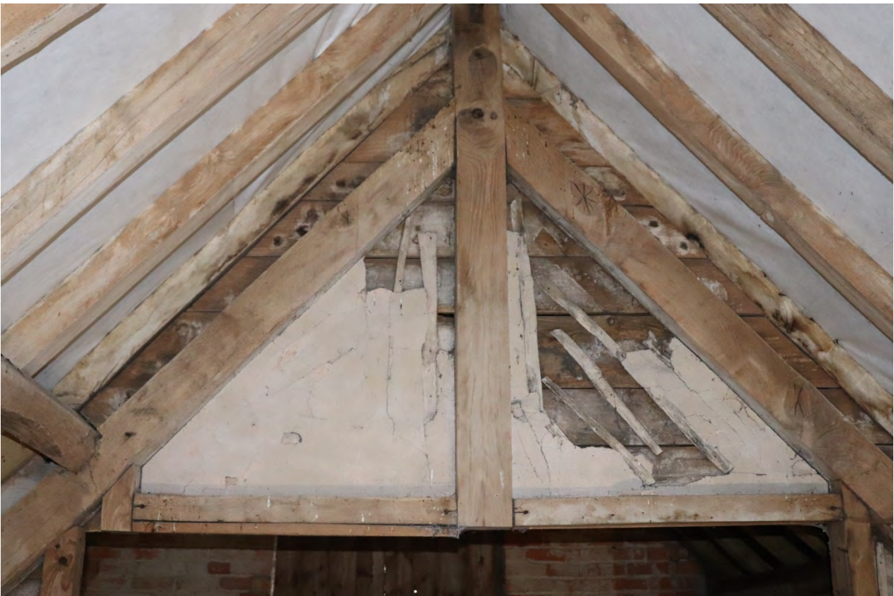
Plate 27 Phase 3 lathe and plaster to the rear of the boarding, looking east
