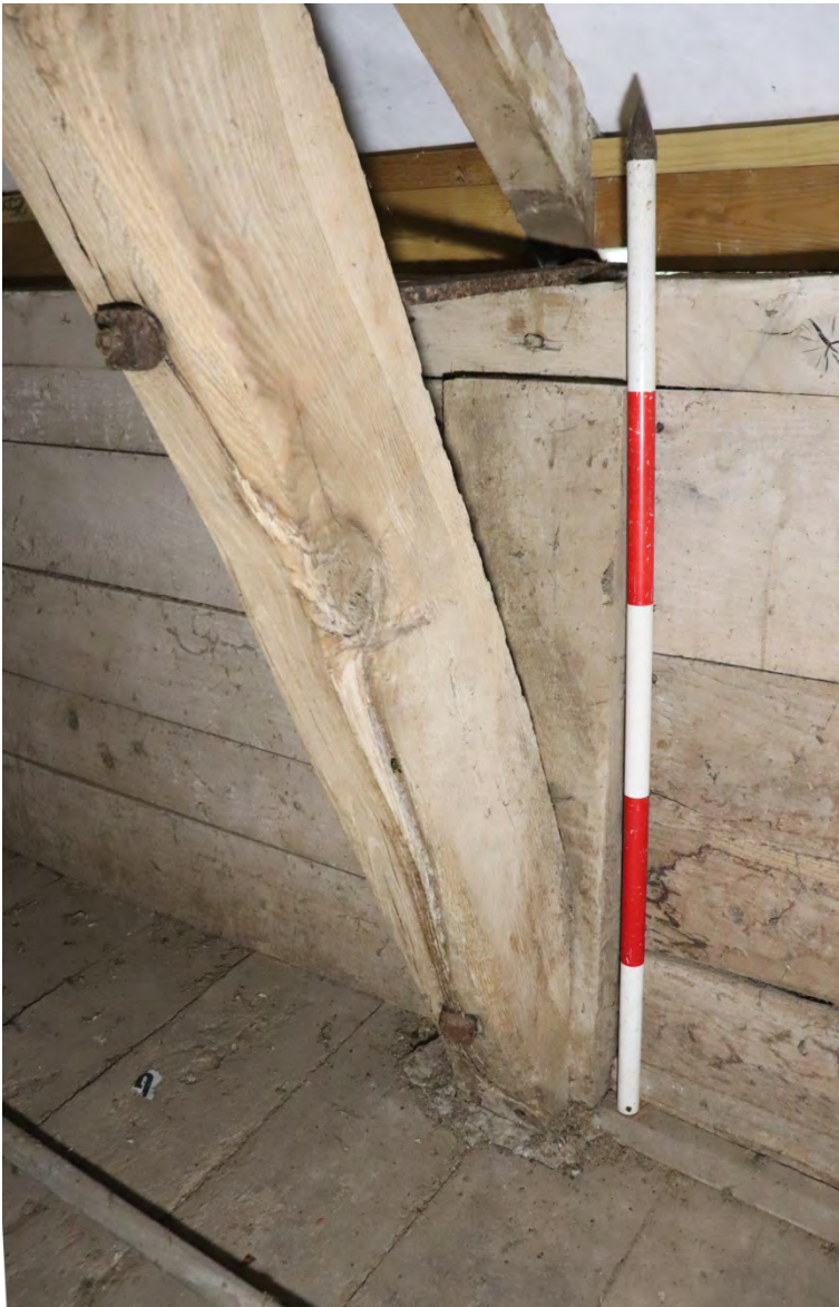
Plate 25 Phase 3 upper cruck base bolted to the post and strapped to the wall plate, looking north-west, scale 1m
