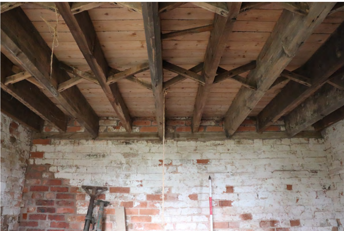
Plate 37 Phase 4 floor with lattice bracing, looking north, scale 0.60m of 2m scale visible
