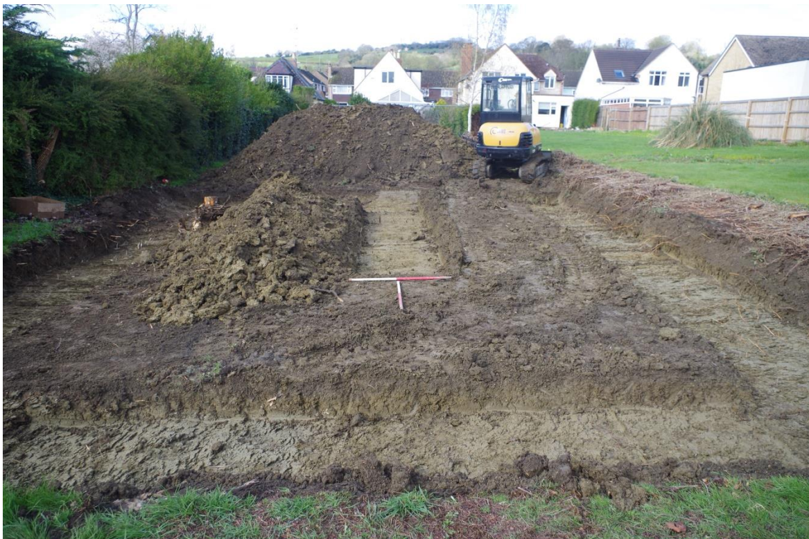
Plate 2: Looking west across the development area. The footings trench has been machined to the natural substrate, 1m scales.
