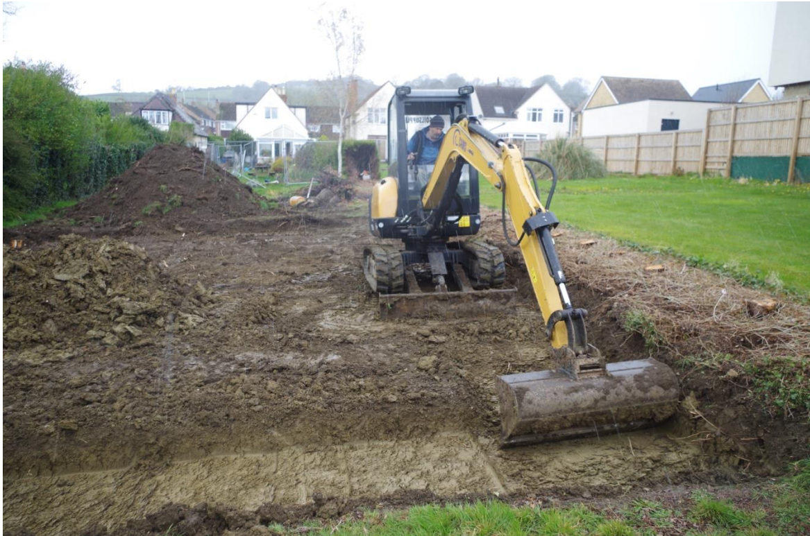
Plate 1: Looking west across the development area, with the machining of the footings trench in progress.
