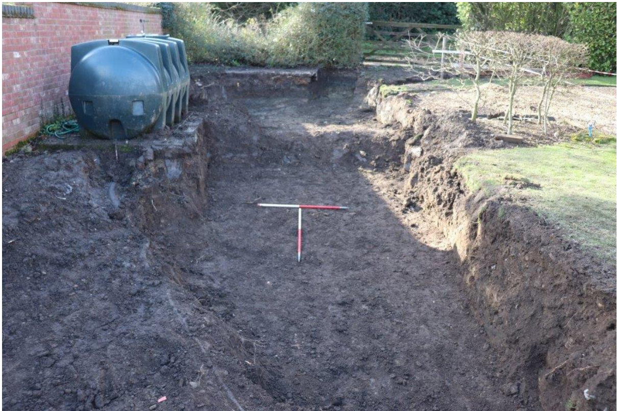
Plate 2: Trench 1 access road groundworks, west end, view west to B4368 road, 2x 1m scales
