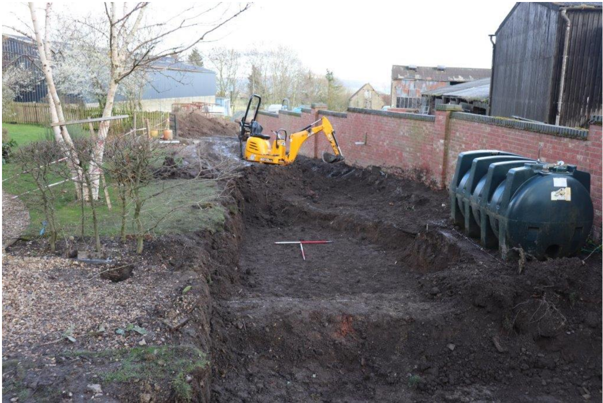
Plate 3: Trench 1 access road, modern oil pipe in foreground, view south-east, 2x 1m scales
