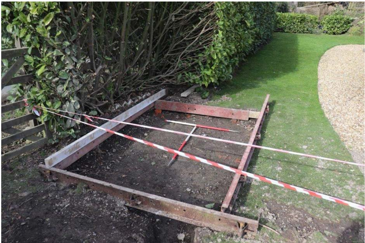
Plate 4: Trench 2 base for new oil tank on north-west side of site, view north, 2x 1m scales
