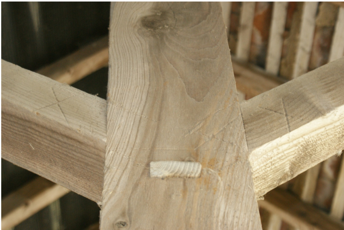
Plate 15 Barn 2, Phase 3 shelter shed, carpenters marks on the roof trusses, numbered from 1-10 in Roman numerals starting with truss number 1 southern end of the building, looking south (no scale)
