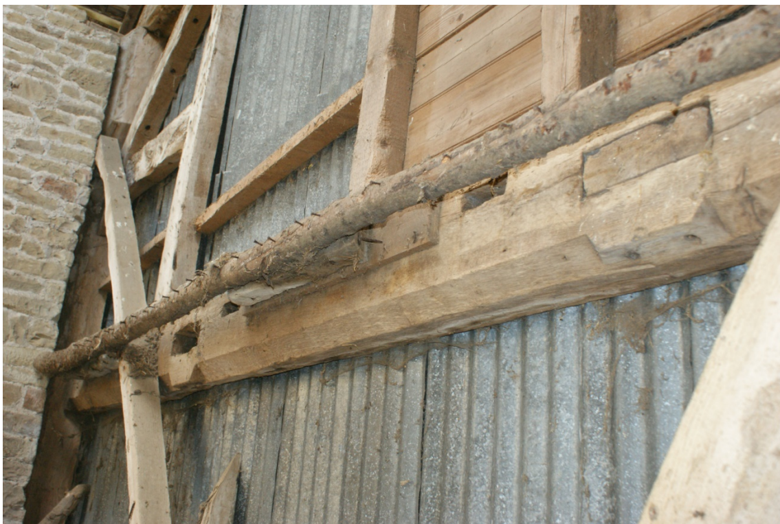
Plate 6 Phase 1 reused domestic floor joist, looking north-east, at north end of Barn 1 (no scale)
