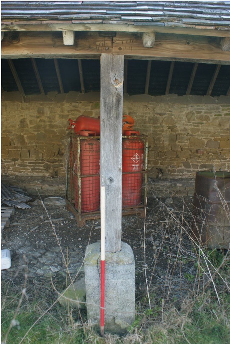
Plate 16 Barn 2, Phase 3 shelter shed, bay post with carpenters marks visible on the wall plate that correspond to the internal roof truss, looking south-east (1m scale)
