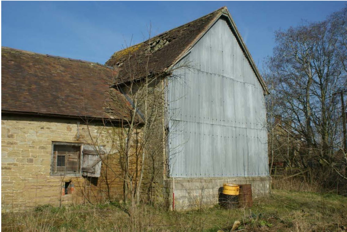
Plate 5 Phase 1 truss position, looking north-west, at north end of Barn 1 (1m scale)
