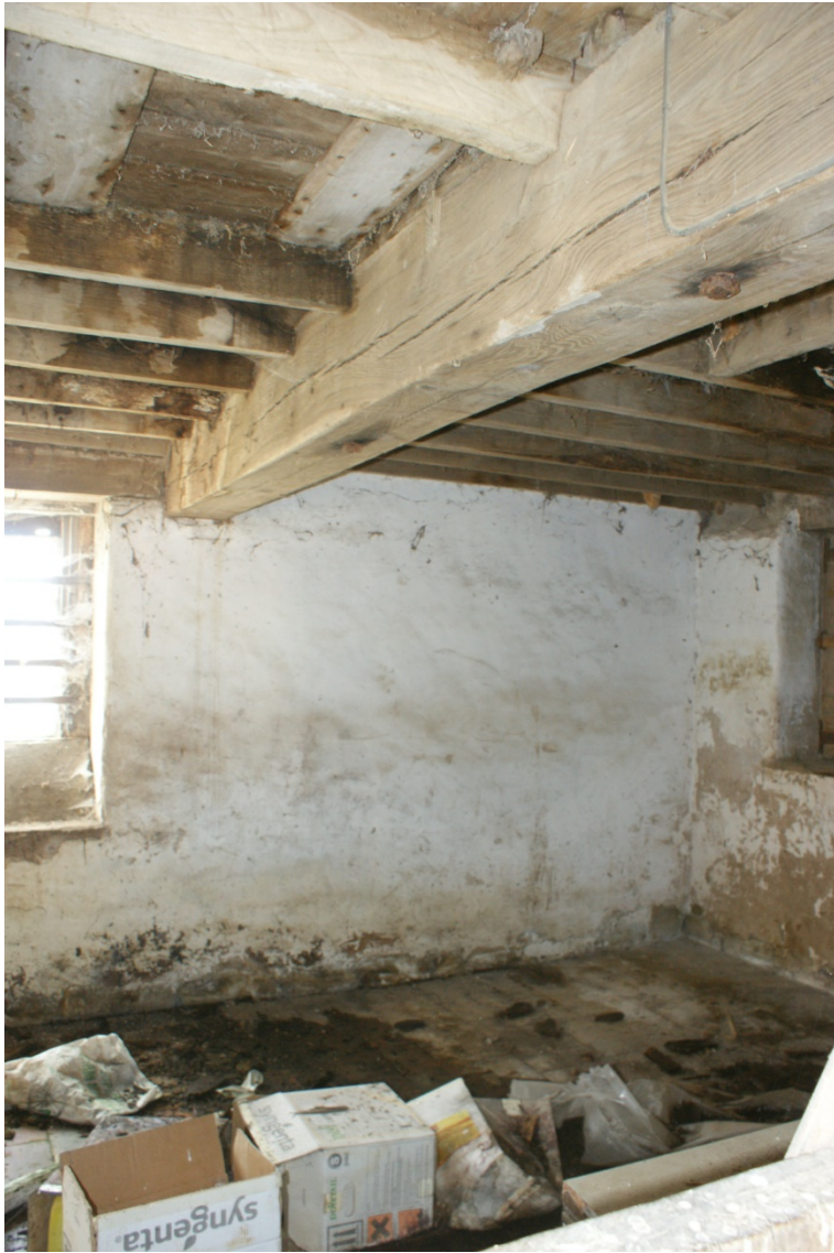
Plate 28 Barn 2, Phase 3 cart shed, stable and storage building, looking south-east (no scale)
