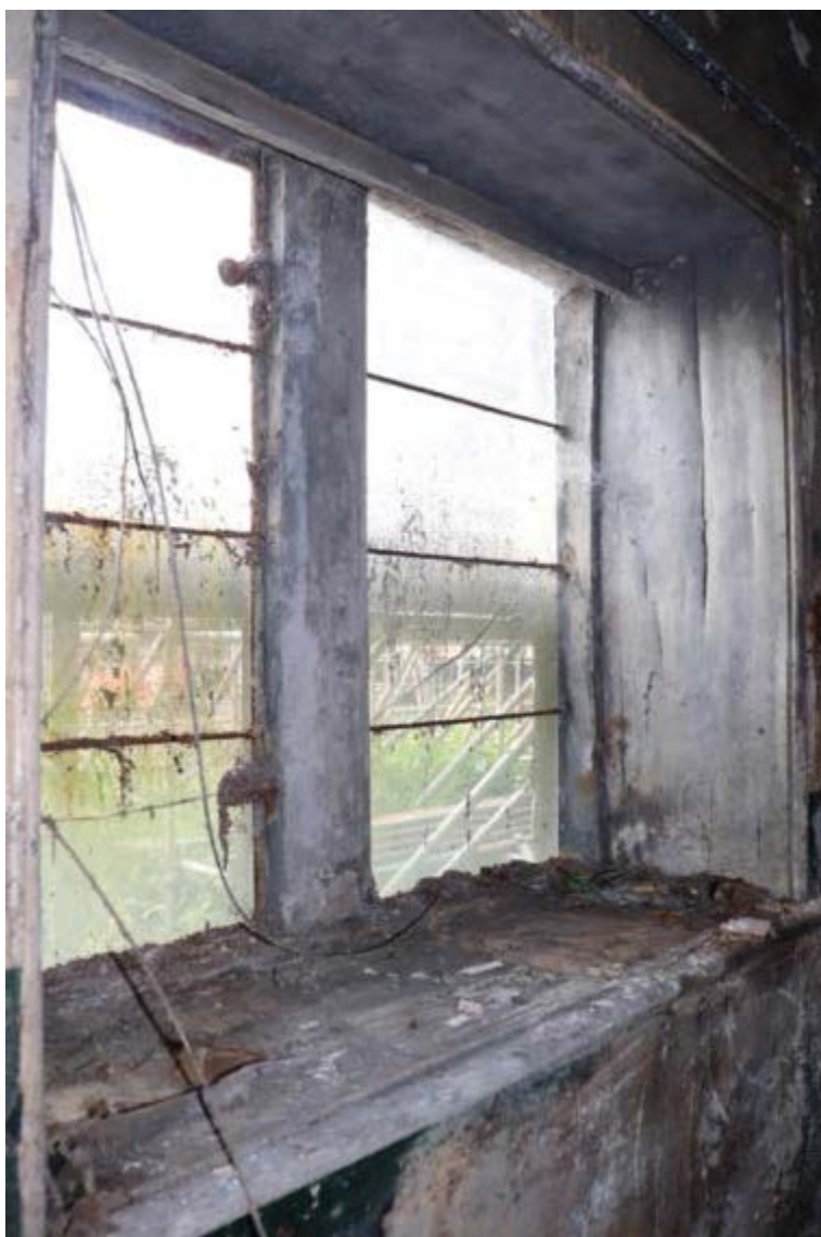
Plate 121 Phase 3 room G17c wooden frames with tie bars demonstrating that they had small pane windows, as shown on Plate 122, looking south, no scale
