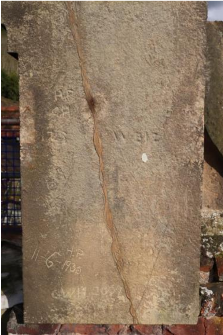
Plate 168 Graffiti on the rear of the parapet above the porch, looking north-west, no scale
