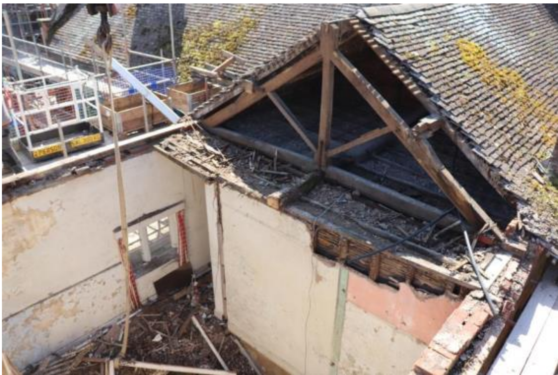
Plate 86 Phase 2 room F16 with Phase 3 roof truss above, looking south, no scale
