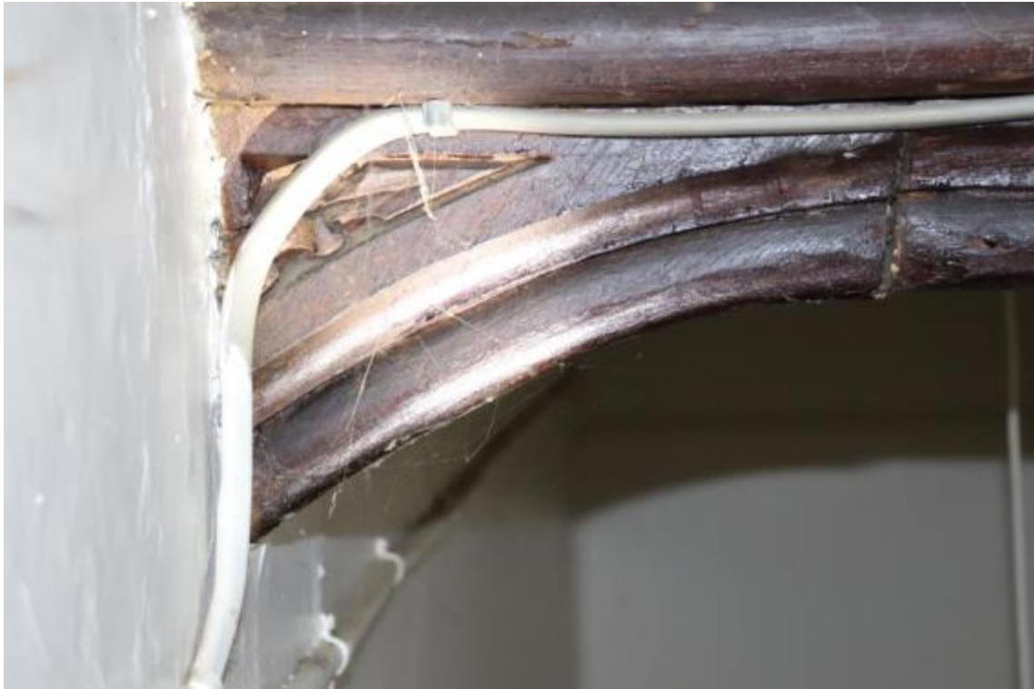
Plate 41 Phase 1 curved bracket beam end with foliate decoration, looking north-west, no scale
