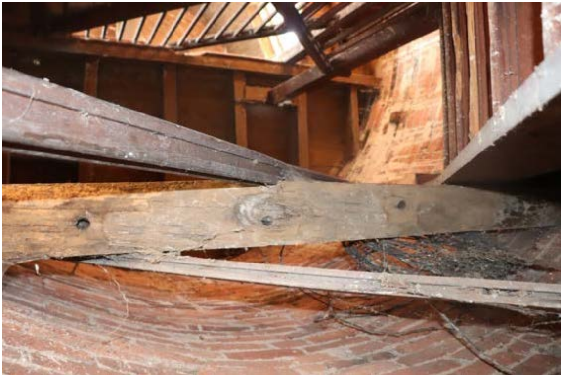
Plate 55 Underside of probable Phase 1 purlin with regular peg holes through what would have been its upper side; see Figure 12 for profile
