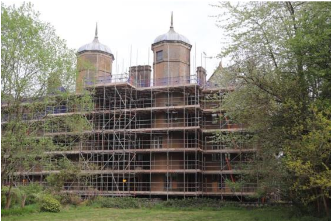
Plate 31 The house looking north towards the Phase 1 element, which was rebuilt in Phase 3, no scale
