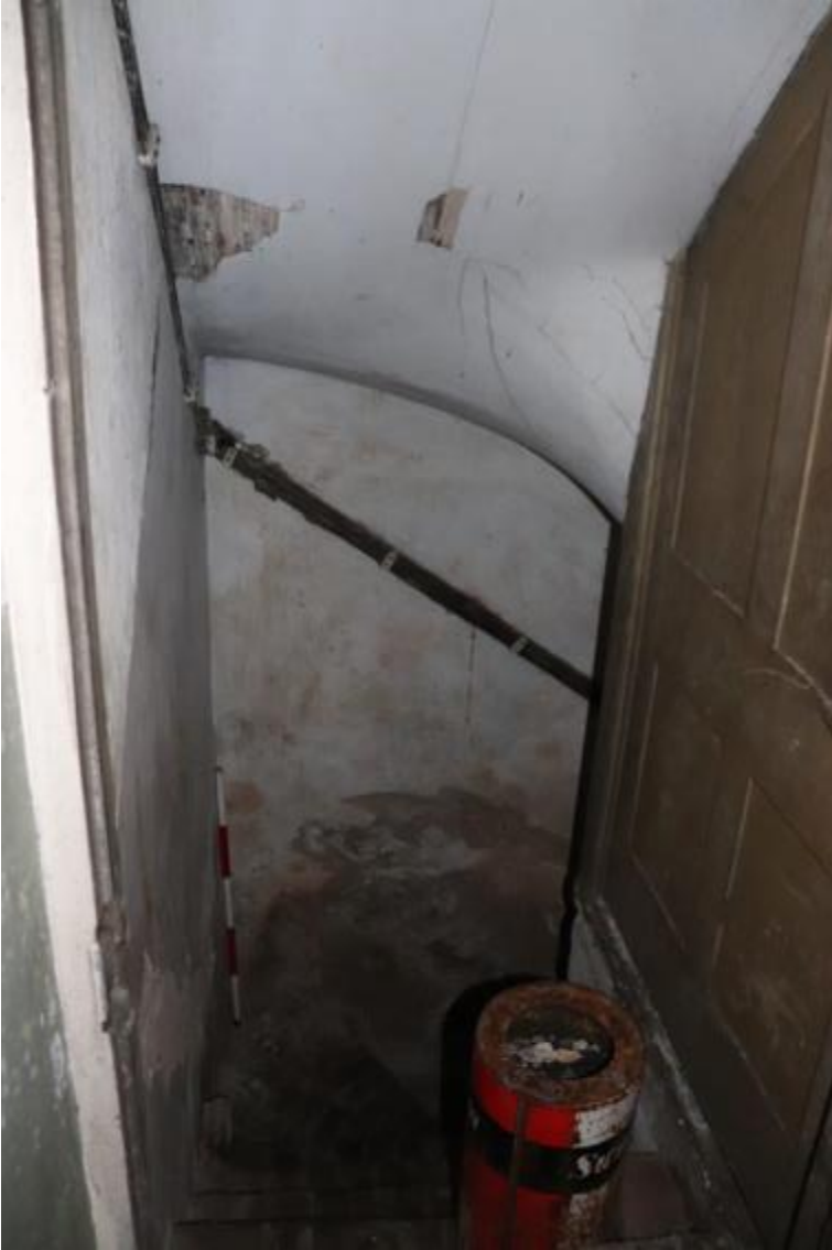
Plate 150 Phase 4 stairs from G11 into the Phase 2 cellar, looking south-east, scale 1m
