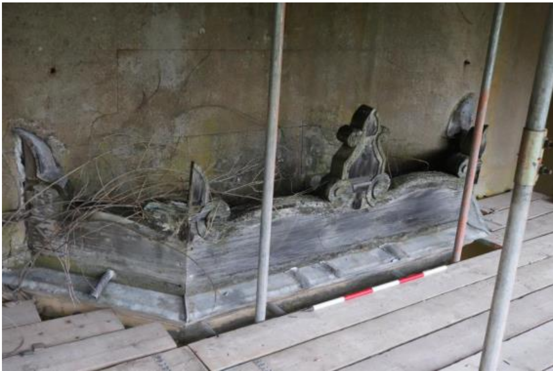
Plate 118 Phase3 timber parapet detailing above the canted oriole window, looking east, scale 1m
