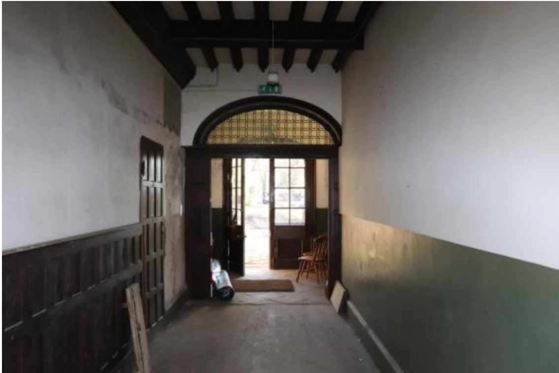
Plate 39 Phase 1 moulded ceiling structures within the house entrance, with Phase 3 above the low arch and Phase 6 panelling and door to the left, looking north-east, scale 1m
