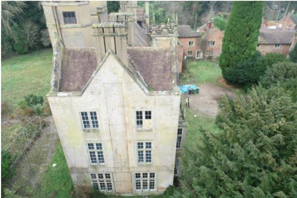
Plate 33 The house with the Phase 1 elements, rebuilt in Phase 3, on the left, and the Phases 2 wing in the background, looking north-west, no scale
