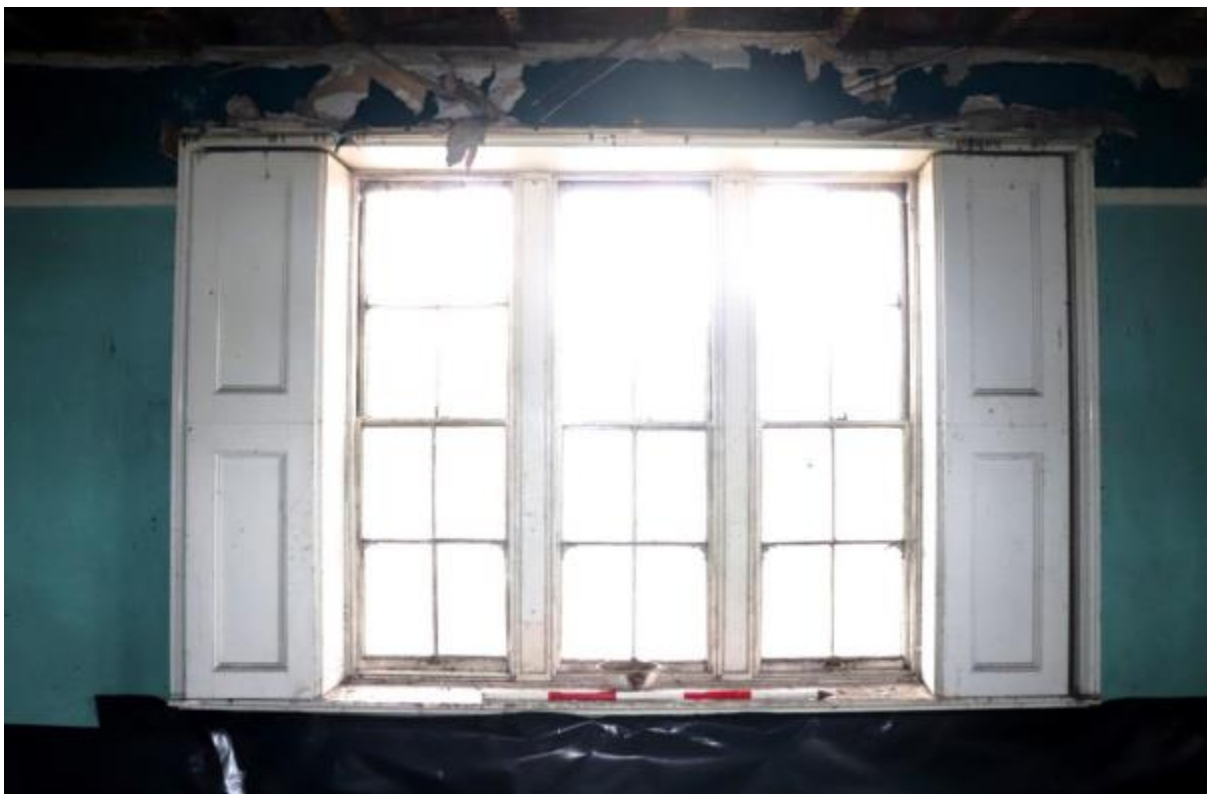
Plate 115 Phase 3 internal window and shutter detail, room S1, looking north-east, scale 1m
