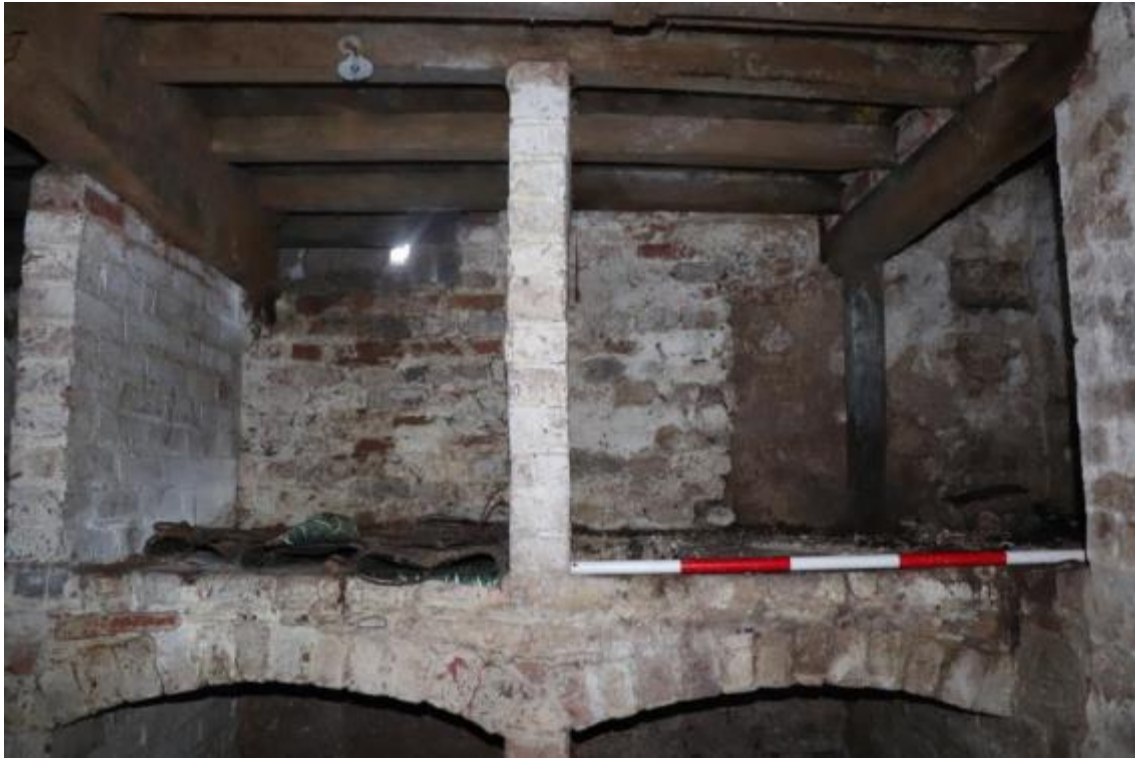
Plate 45 Phase 1 cellar with a blocked opening on the external wall behind later shelving, looking south-west, scale 1m
