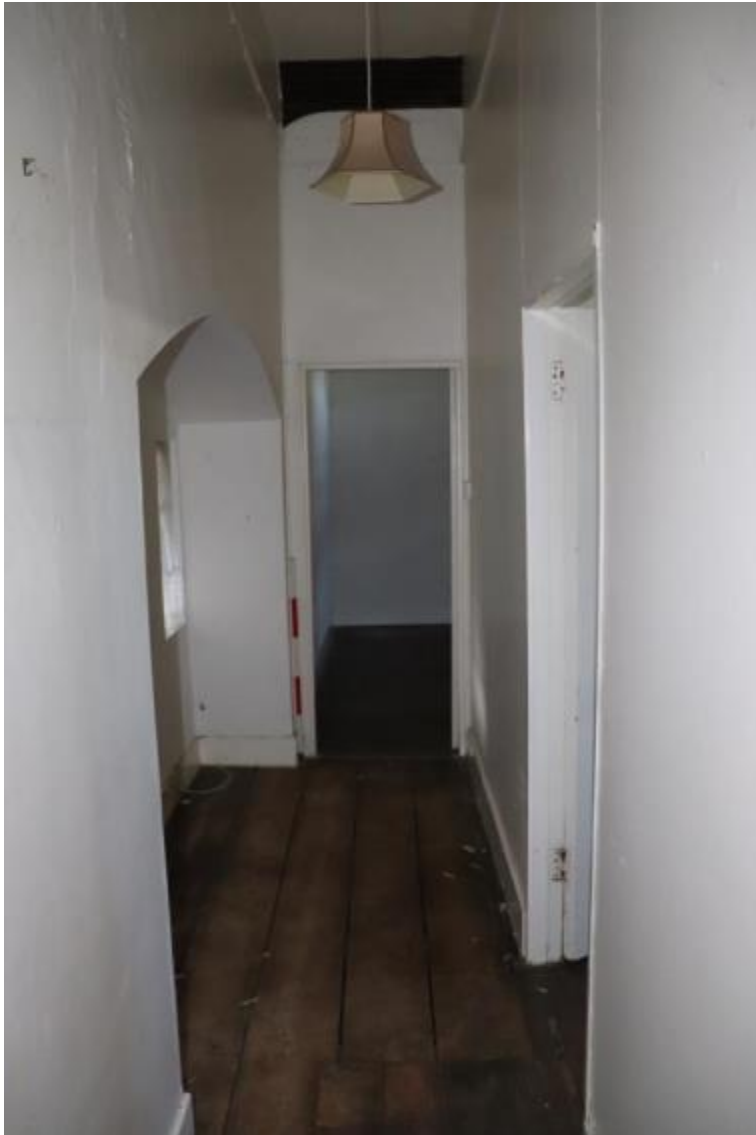
Plate 42 Corridor on the south side of room G2, with the opening on the left probably the Phase 1 fireplace position, looking north-west, scale 1m
