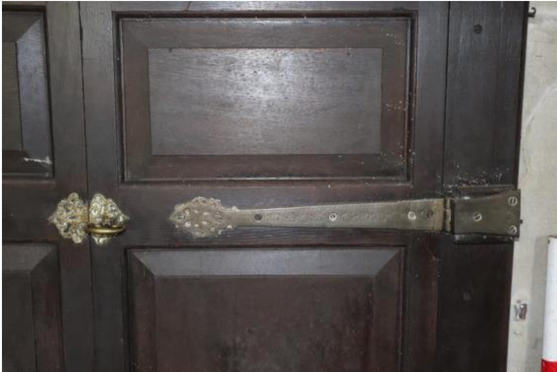
Plate 162 Brass fittings retro fitted in Phase 6, looking north-east, 0.20m scale visible
