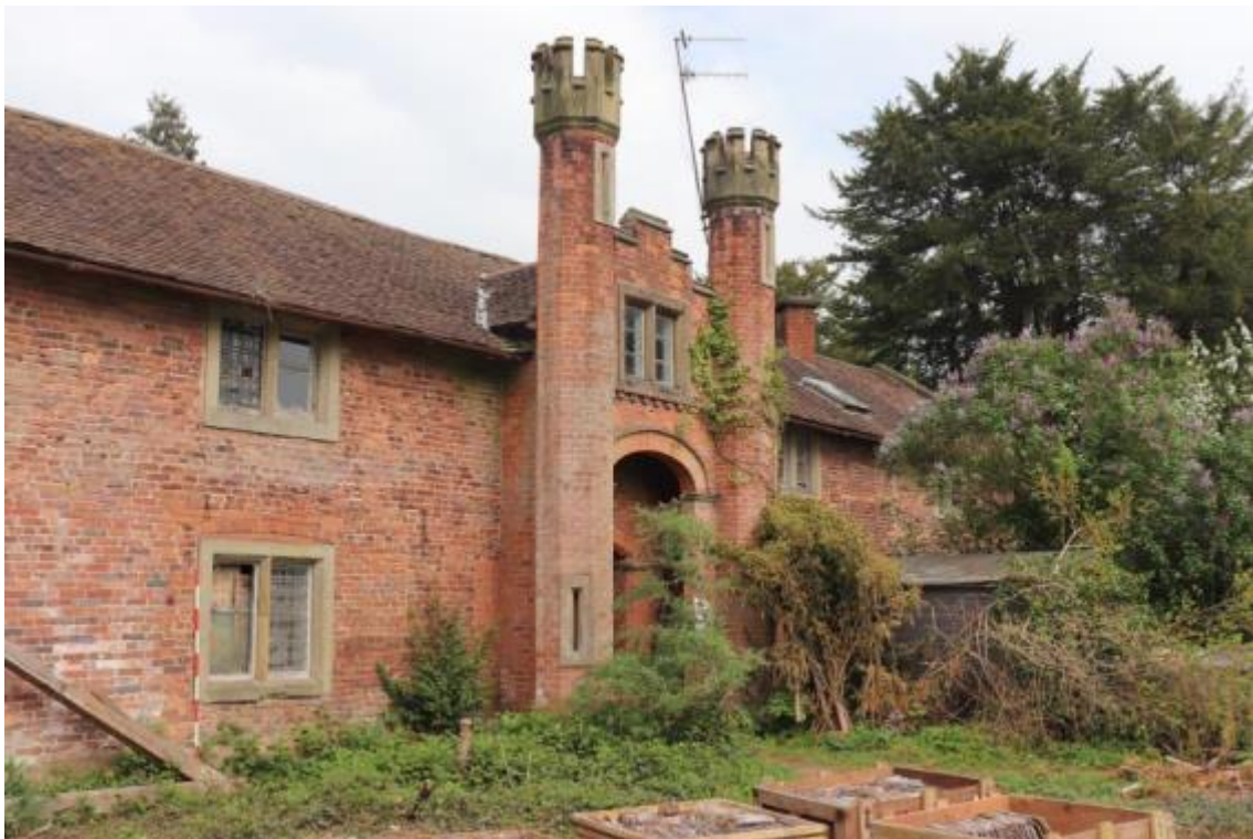
Plate 37 Looking north towards the Phase 2 and later wing and Phase 5 decorative towers, no scale
