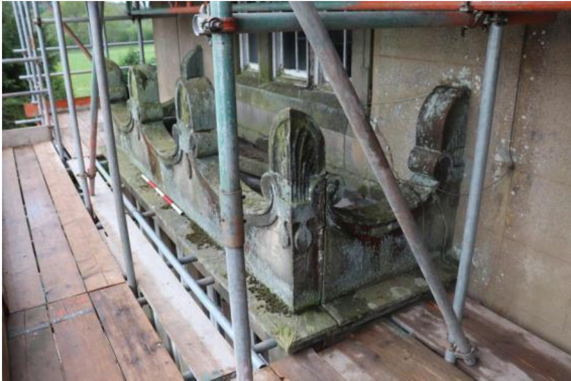
Plate 119 Phase 3 stone parapet detailing above the projected bay window, looking south, scale 1m
