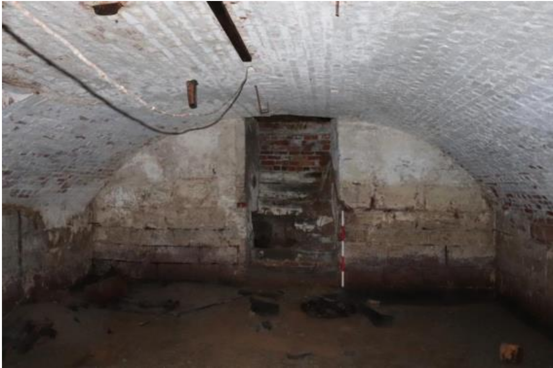
Plate 74 Phase 2 cellar with stairs into the kitchen above, looking north-west, scale 1m
