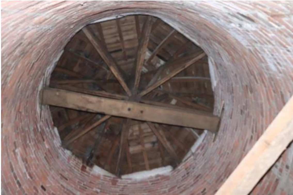
Plate 54 Interior of the northern turret, with only Phase 3 fabric visible, looking upwards to the roof structure
