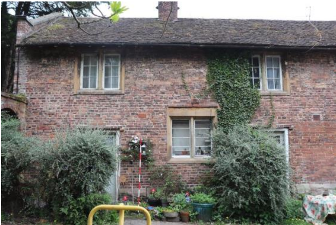
Plate 123 Phase 3 wood frame casement windows added to the north-west facing elevation of the Phase 2 building, see here on the first floor, looking south-east, scale 2m
