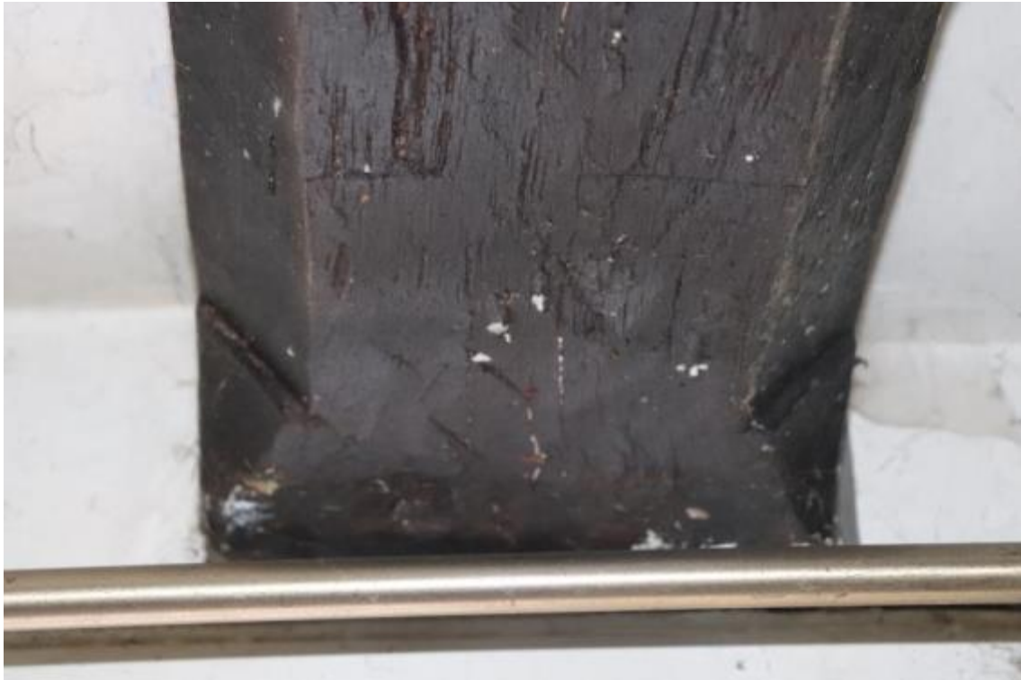
Plate 104 Phase 2 beam end chamfer in room G23, looking north-west, no scale
