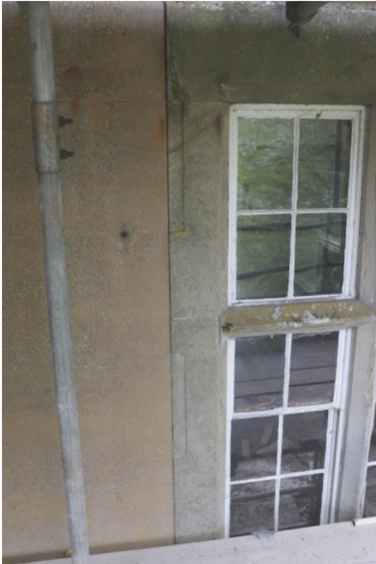
Plate 120 Phase 3 carved indent on window frames, matching the alignment of the stone effect lines within the mortar of the walls, no scale
