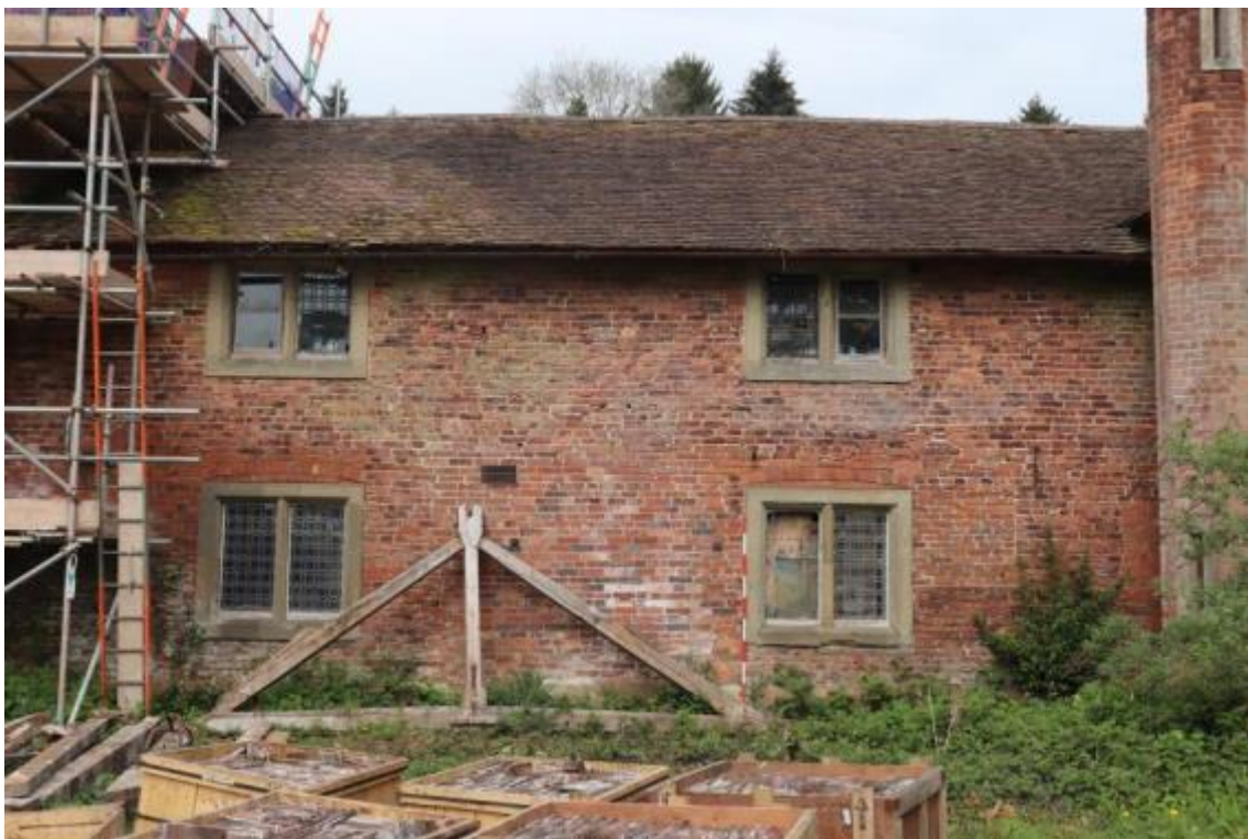
Plate 94 Phase 2 blocked wide doorway, looking north-west, with removed Phase 3 King Post, scale 2m (see Figure 14 for reconstruction)
