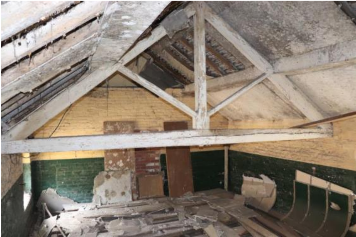
Plate 93 Phase 2 room F19 with Phase 3 roof truss above, looking north-east, no scale
