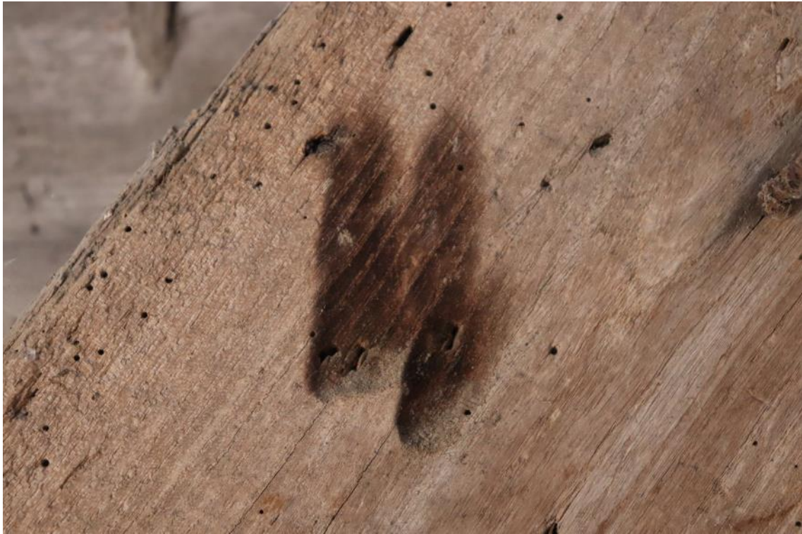
Plate 18 Candle burn marks on Truss 3, looking south, no scale
