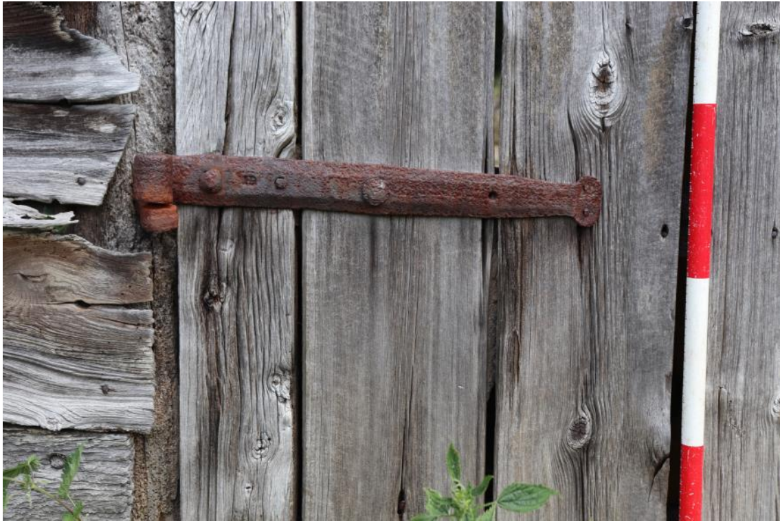
Plate 10 Phase 2 barn exterior original door hinge, looking east, each scale element is 0.20m
