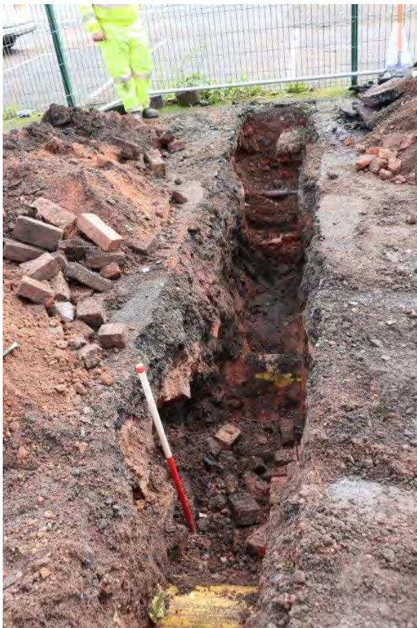
Plate 4: Cellar structures and modern backfill, cut by modern services in Trial Pit 2, view south, 1m scale
