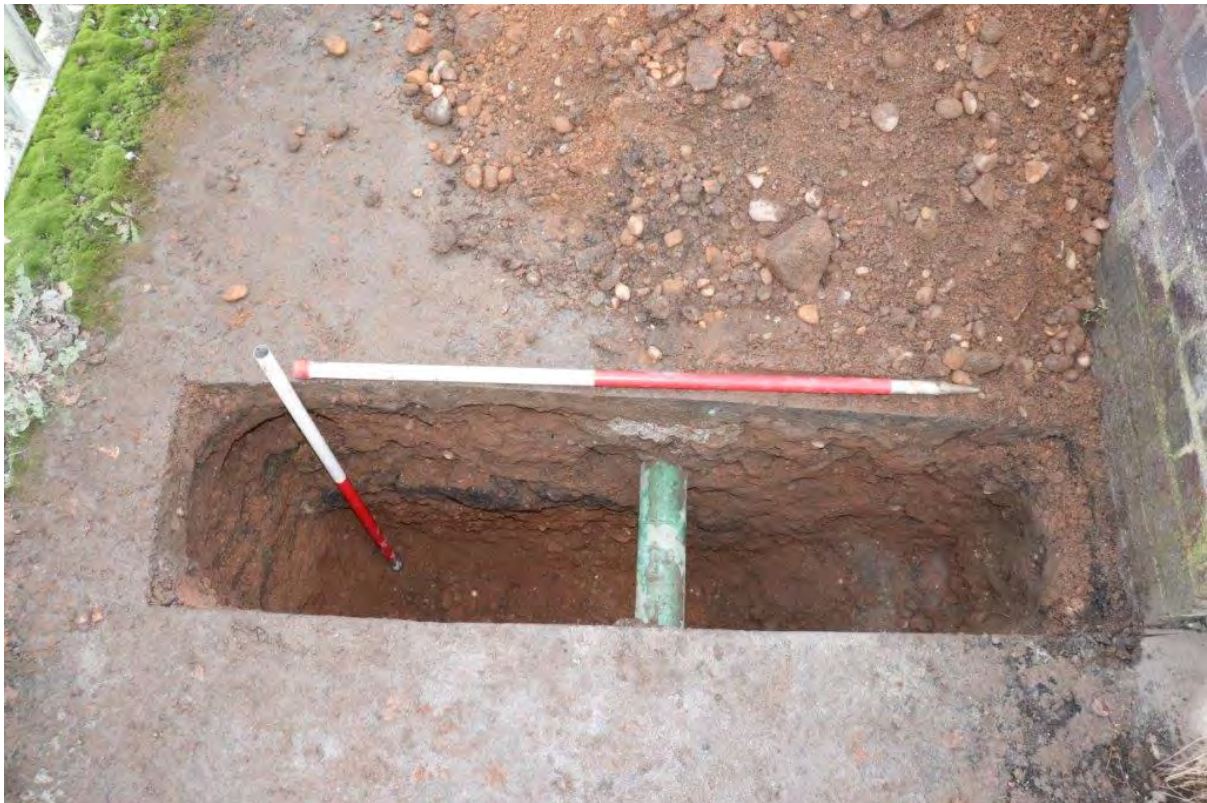
Plate 11: Trial Pit 8 showing modern services and backfill, view west, 2x 1m scales
