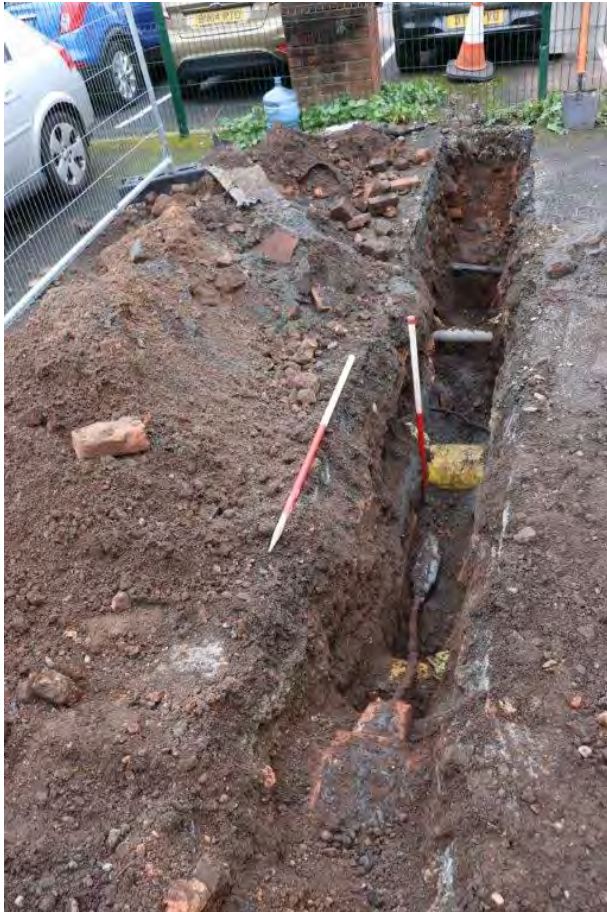
Plate 5: Cellar walls and modern backfill in Trial Pit 3, cut by modern services, view south, 2x 1m scales
