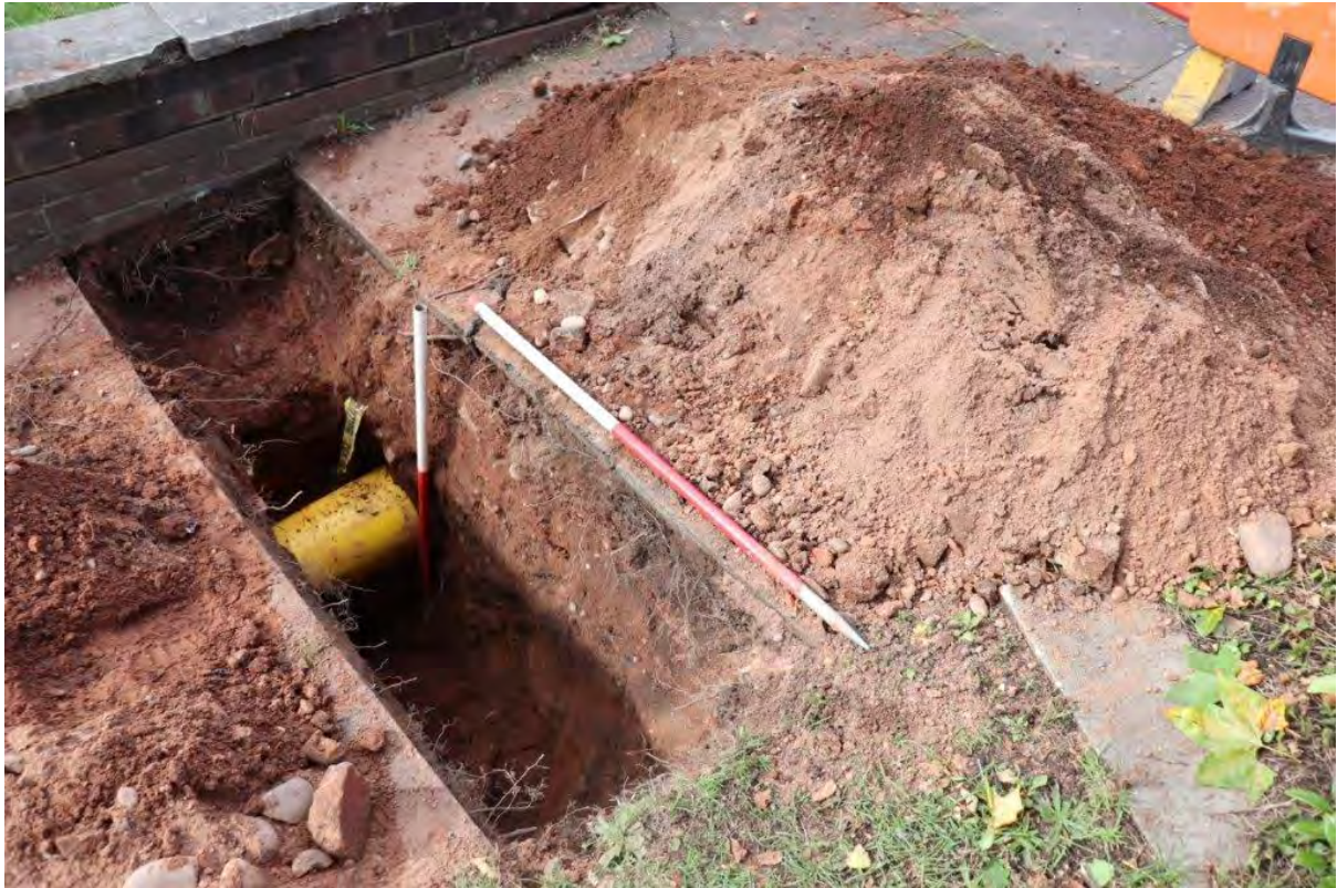
Plate 9: Trial Pit 6 showing modern services and backfill, view west, 2x 1m scales
