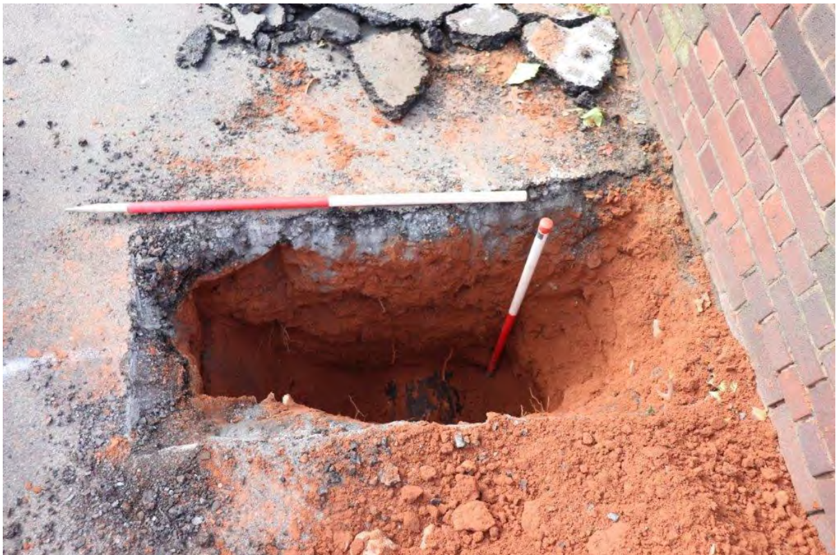
Plate 10: Trial Pit 7 showing modern services and backfill, view west, 2x 1m scales
