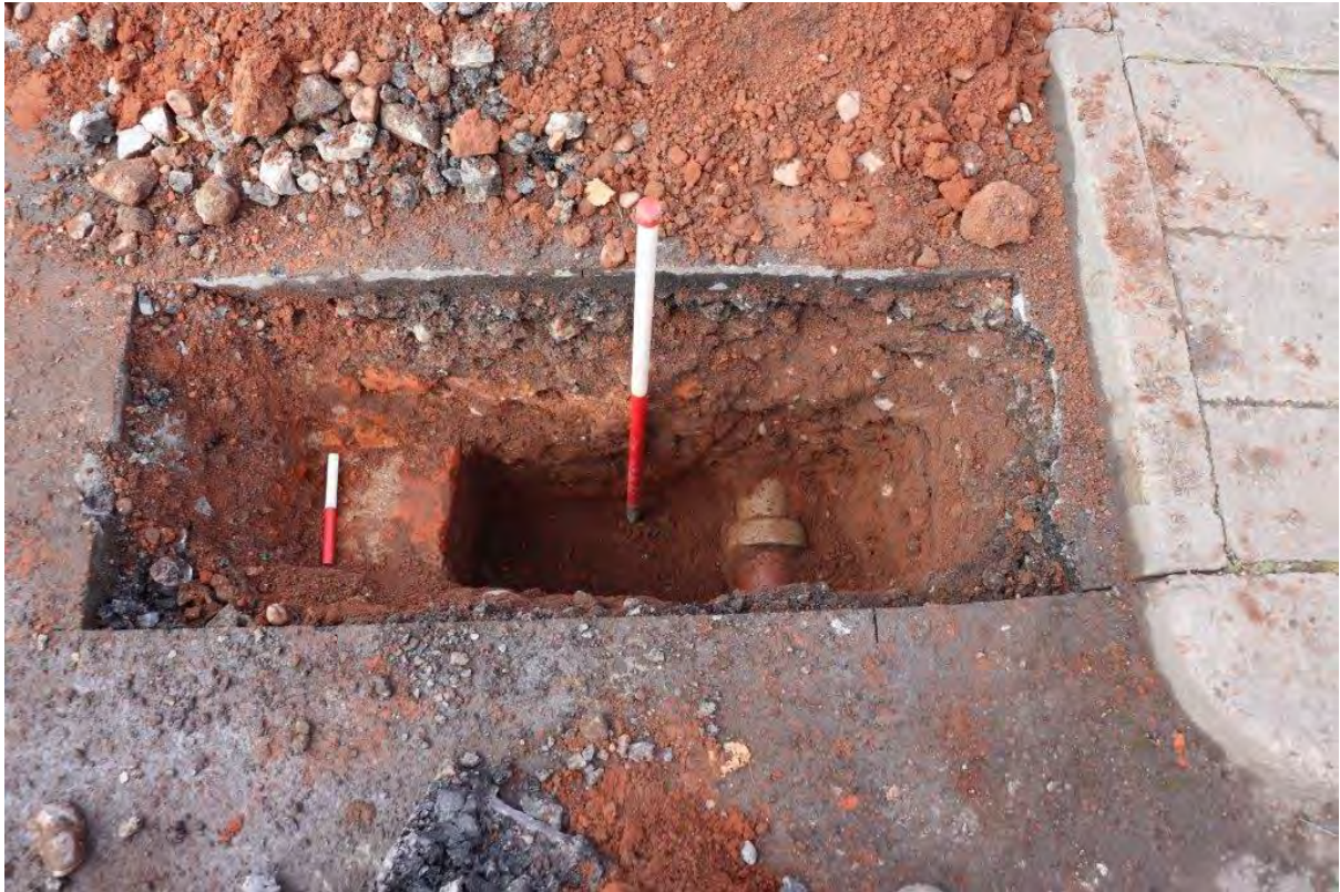
Plate 7: Brick wall in Trial Pit 11, with modern service to east, view north, 0.2m and 1m scales
