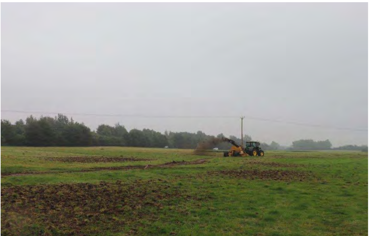
Plate 2: General view of the tractor and rotary ditcher excavating a swale, view south-east, no scales
