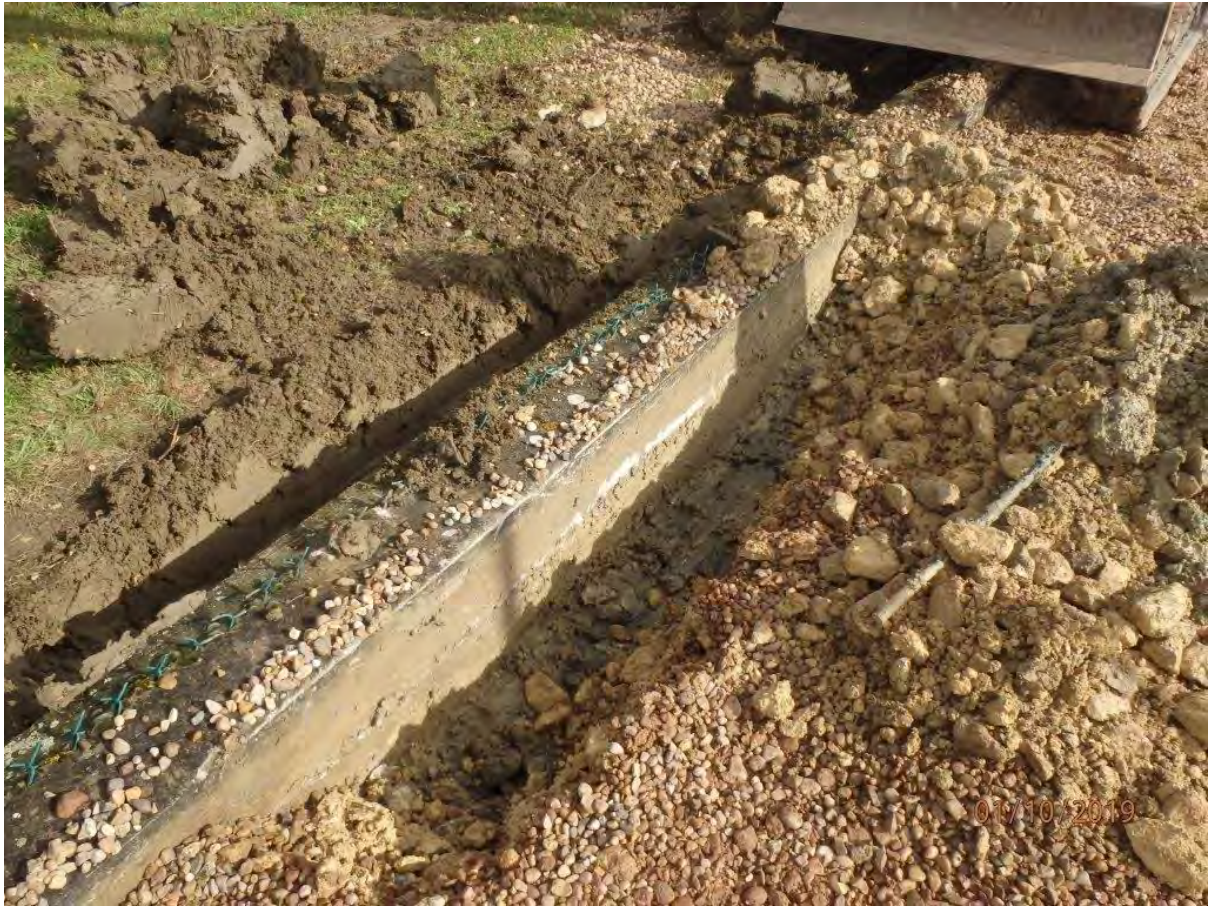
Plate 7: Existing perimeter fence removal, showing extent of concrete foundations, view north-east, no scales
