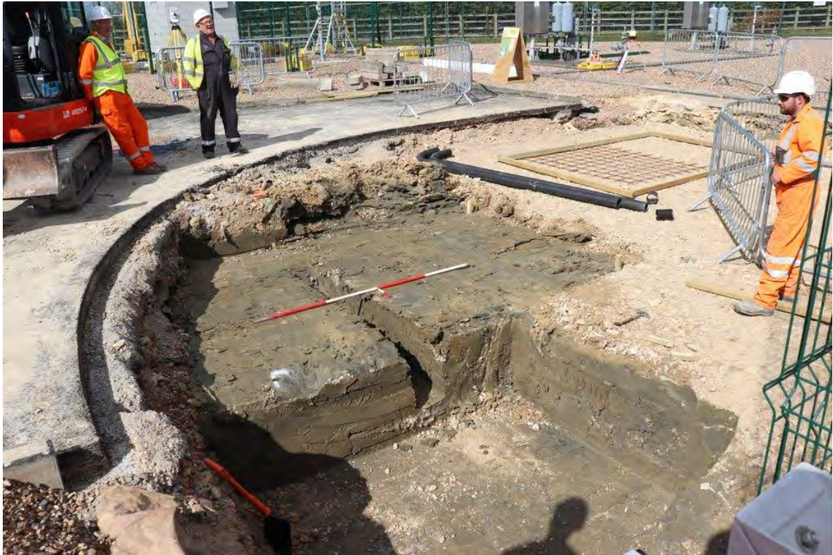
Plate 5: Trench 3 showing modern made ground and natural grey clay, view north, 2m scale
