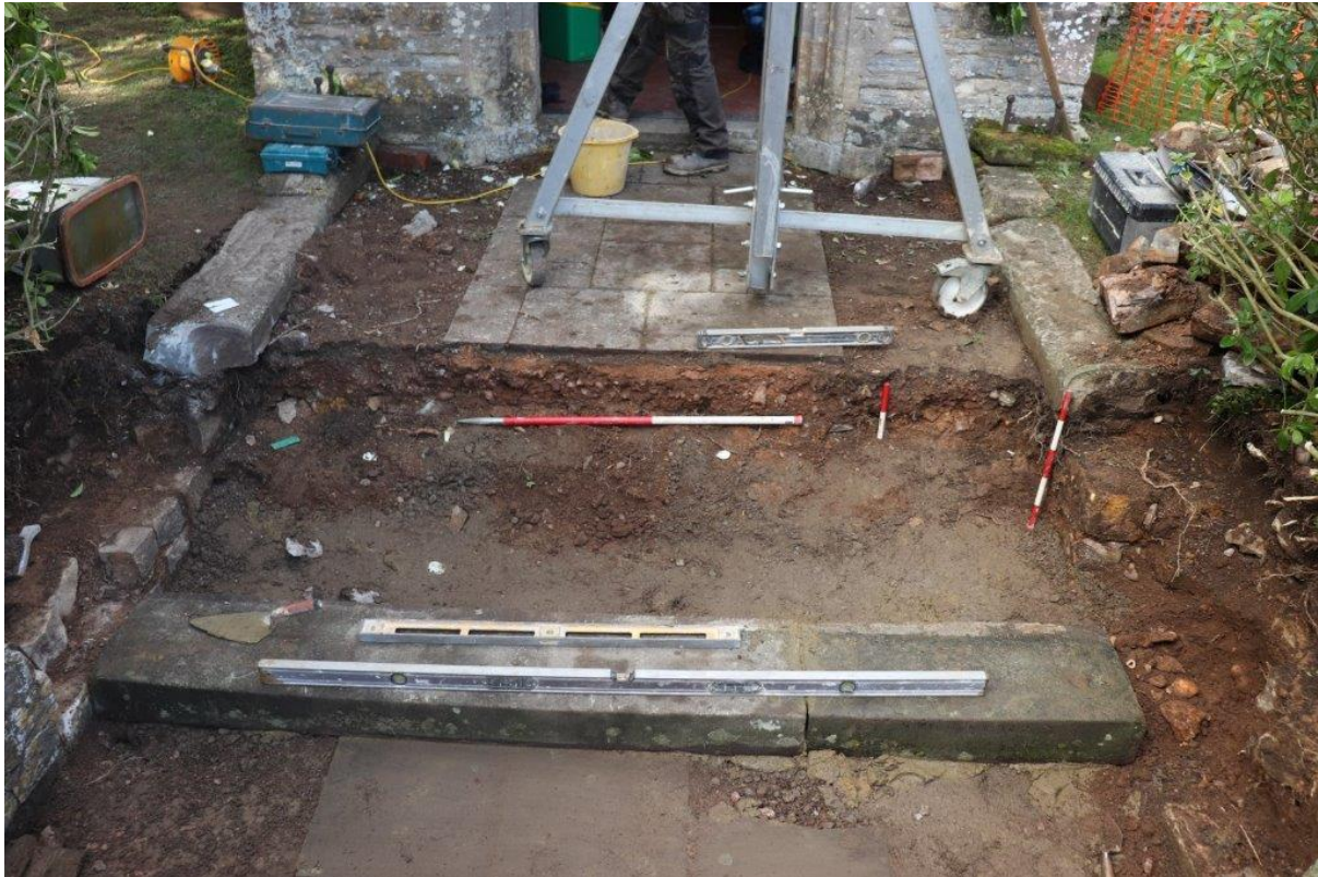
Plate 11: The area of intrusive works following lifting of the steps, showing gravel bedding. 1m, 0.5m and 0.2m scales. View north
