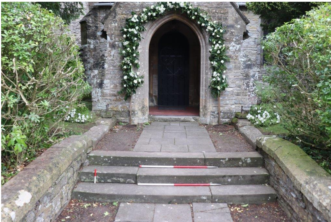
Plate 2: Church steps prior to replacement. 2x1m scales and 0.2m scale. View north
