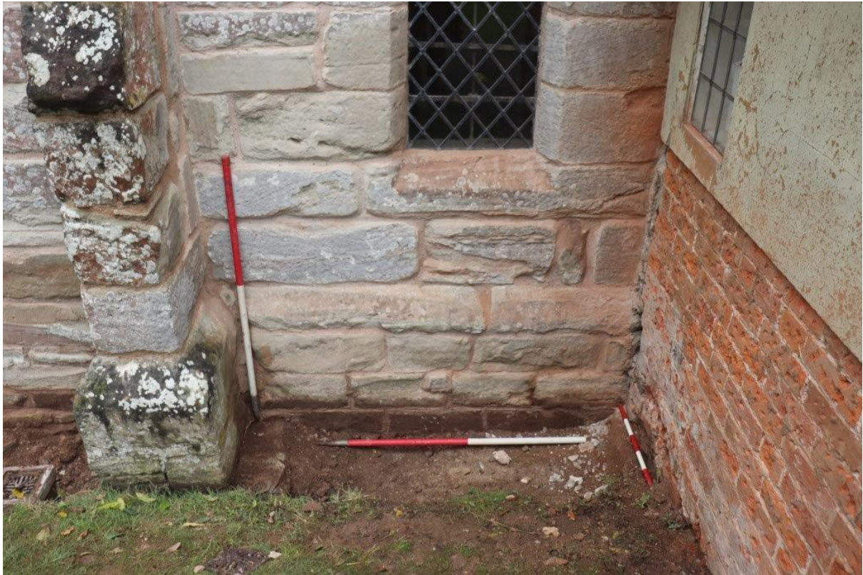
Plate 9: Trench adjacent to the porch, looking North with 1m and 0.5m scales
