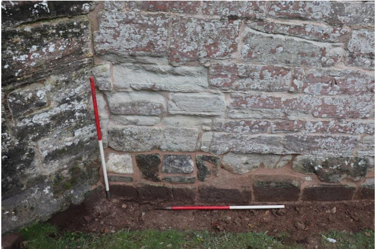
Plate 11: Example of the trench on the South side of the bell tower. 1m scales looking North
