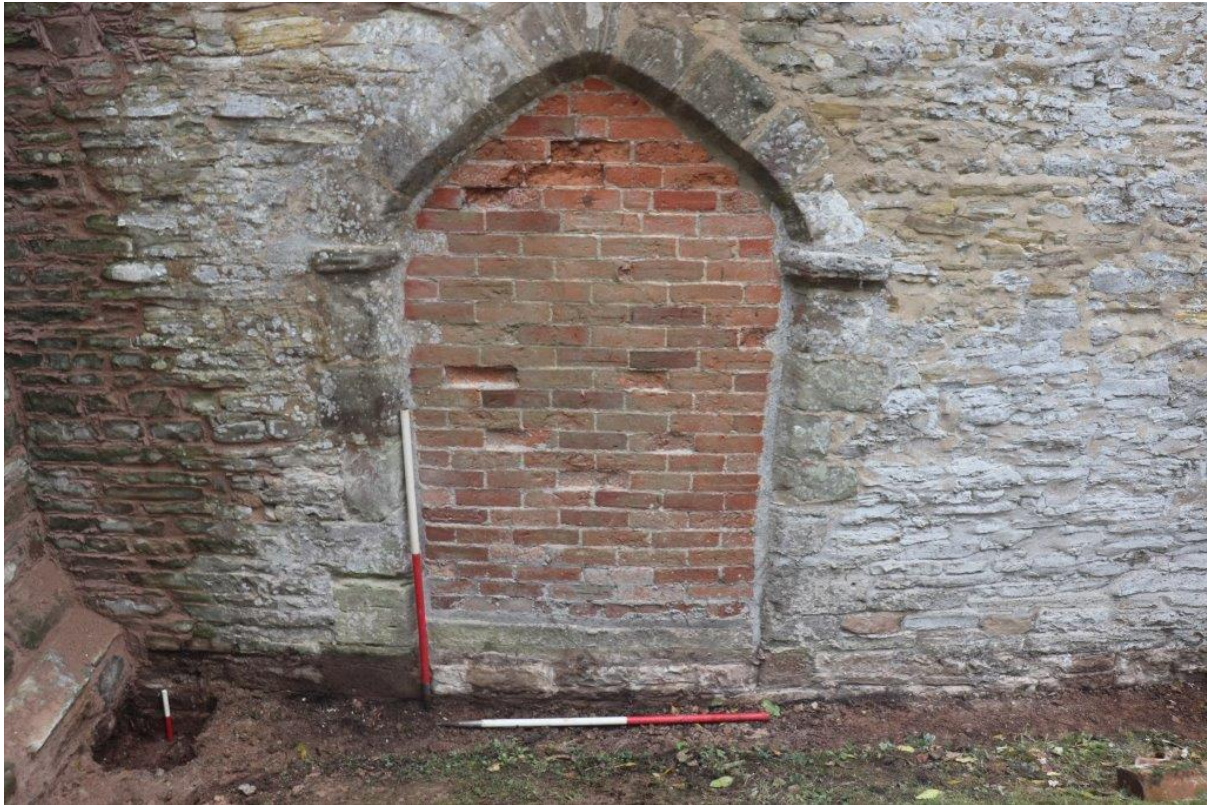
Plate 5: Blocked doorway and trial hole on west side of north transept. 1m and 0.2m scales. Looking South
