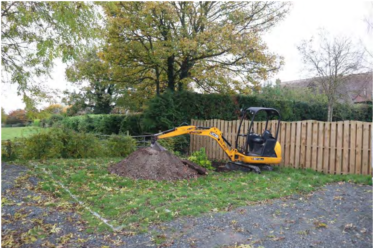
Plate 2: Area of garage foundations at start of excavation (Trench 2), view south-east, no scales
