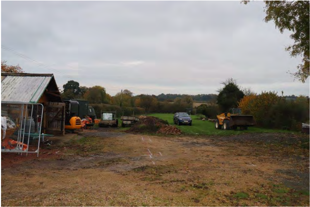
Plate 1: Area of new house foundations prior to excavation (Trench 1), view north, no scales
