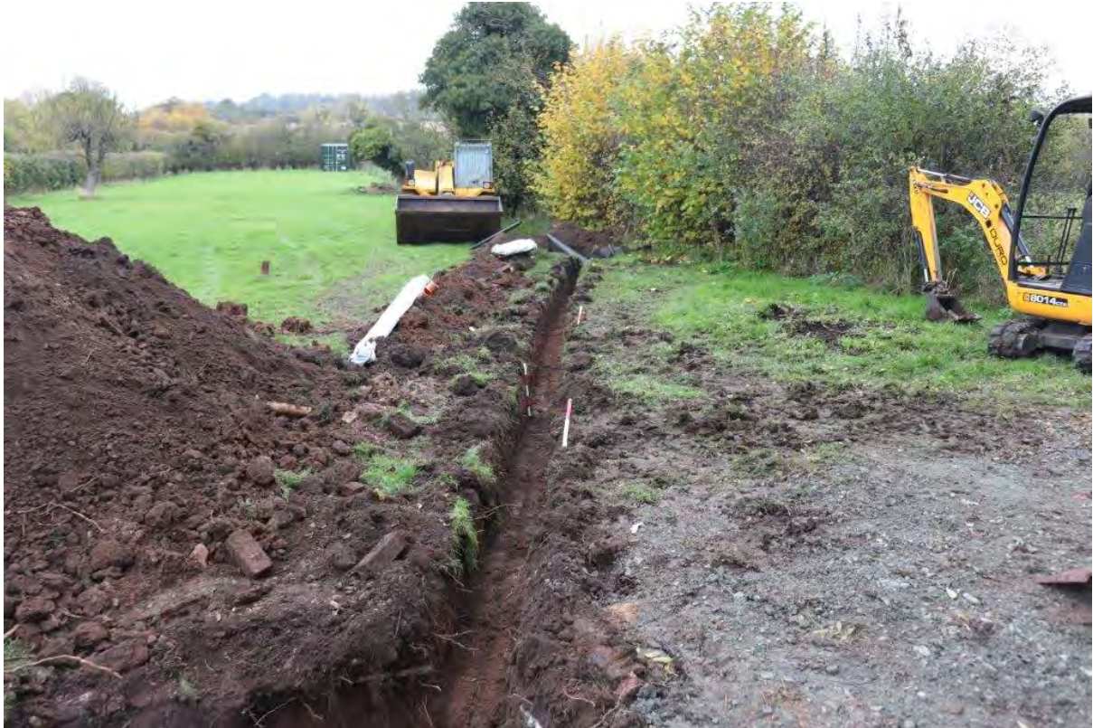
Plate 7: Drainage run and soakaway chamber (Trench 3), view north-east, 0.5m and 2x 1m scales
