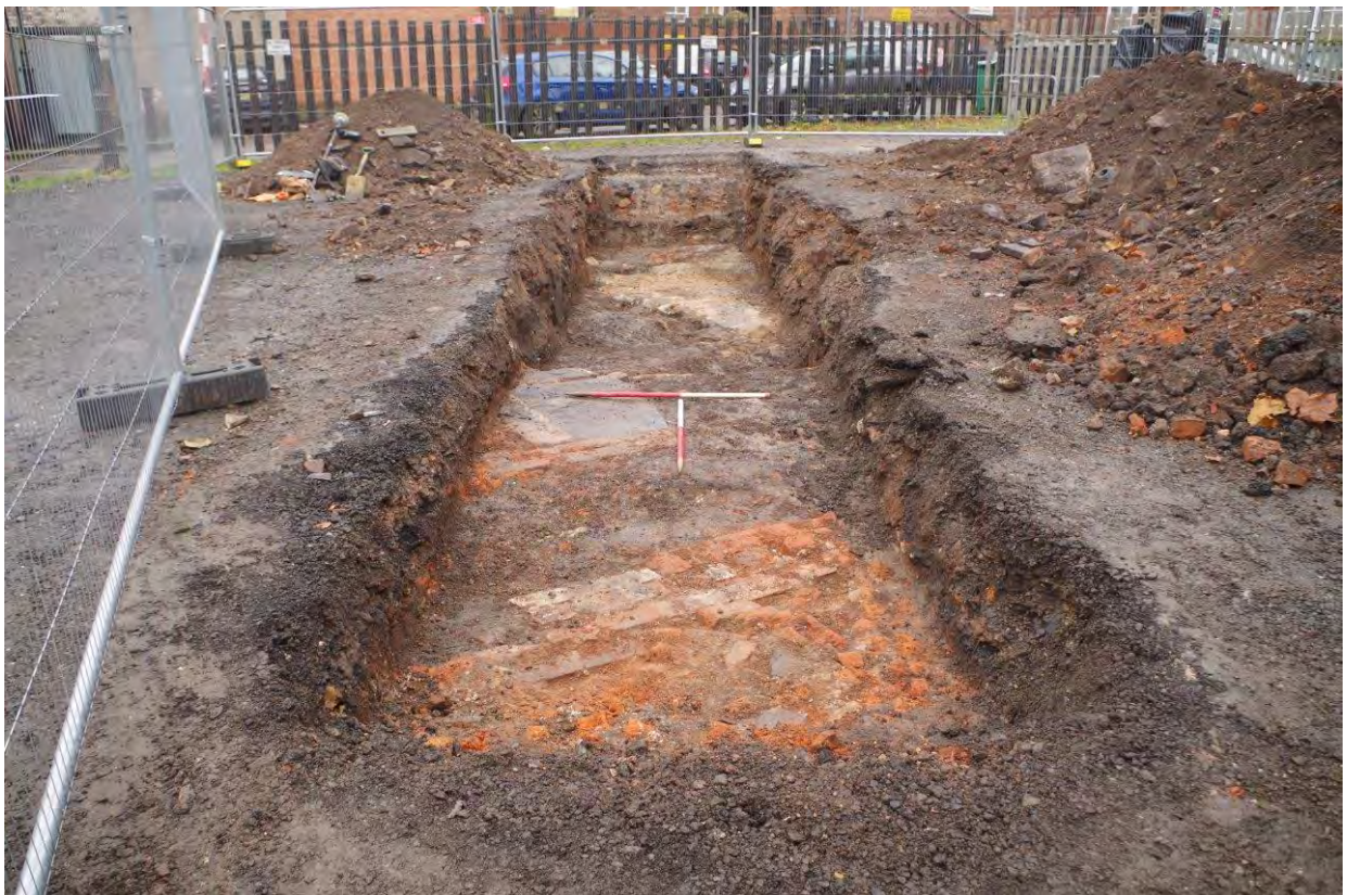
Plate 2: Trench 3, brick walls and surfaces relating to St Georges School, 1m scales, view south-west
