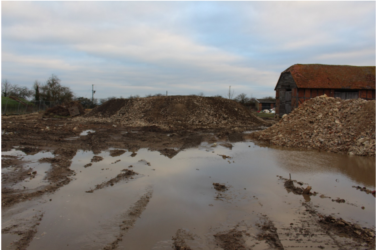
Plate 1: General view of site conditions, looking north, with 17th century barn in background
