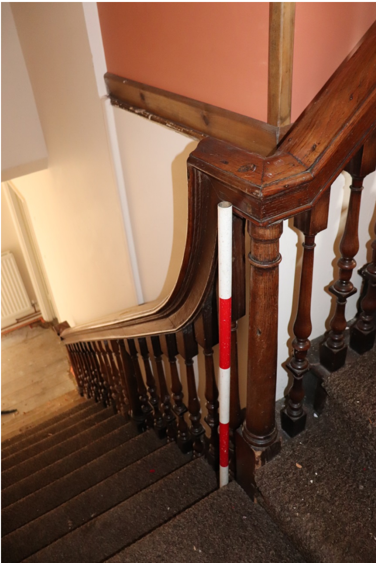
Plate 16 The house ground to first floor stairwell, looking south west, scale 1m
