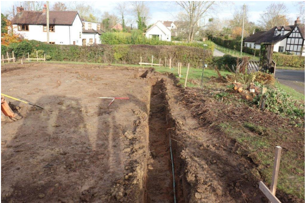
Plate 6: Eastern footing trench showing modern water pipe. Looking north with 1m scales
