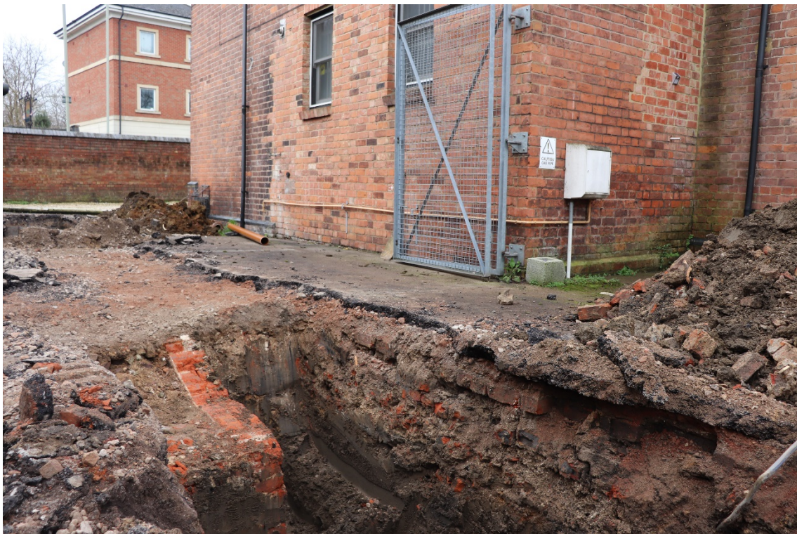
Plate 4: Cellar wall 204 (lower left) was located at the southern end of Trench 2. Note the mortar visible on the inside (left face) of the cellar wall. Photo looking south-west
