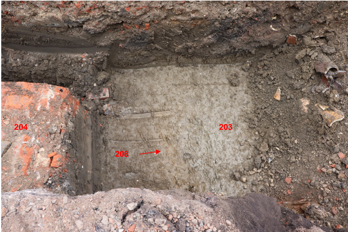
Plate 5: A possible construction cut 208 for cellar wall 204 (left of shot) was observed cut the relict soil (203) (right of shot). A faint orange band in 203 is also visible. Photo looking west
