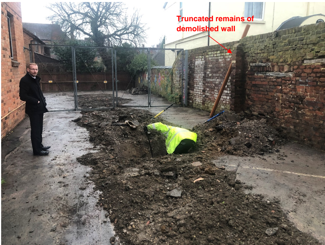
Plate 6: The truncated remains for the demolished wall for the structure visible on historic maps survives as the property boundary. Photo looking north
