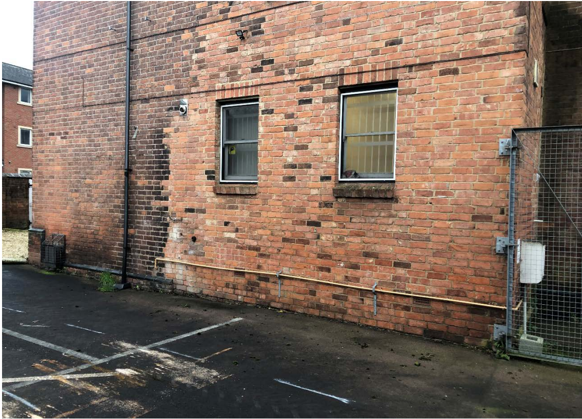
Plate 1: A modern external wall is clearly visible where part of Peter Scott House has been demolished. Photo looking south-west
