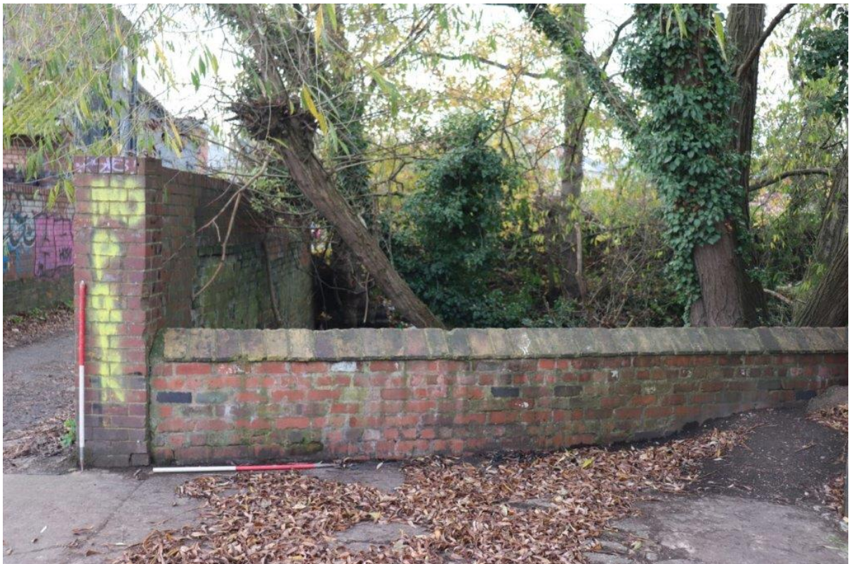
Plate 16: Brick wall with coping stones on north-east side of bridge, view south, 1m scales
