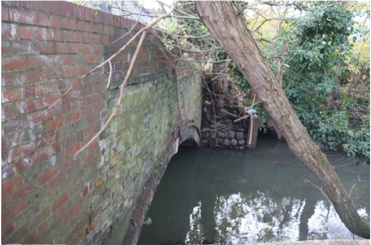
Plate 17: Western side of bridge arch, view south towards modern culvert on southern bank
