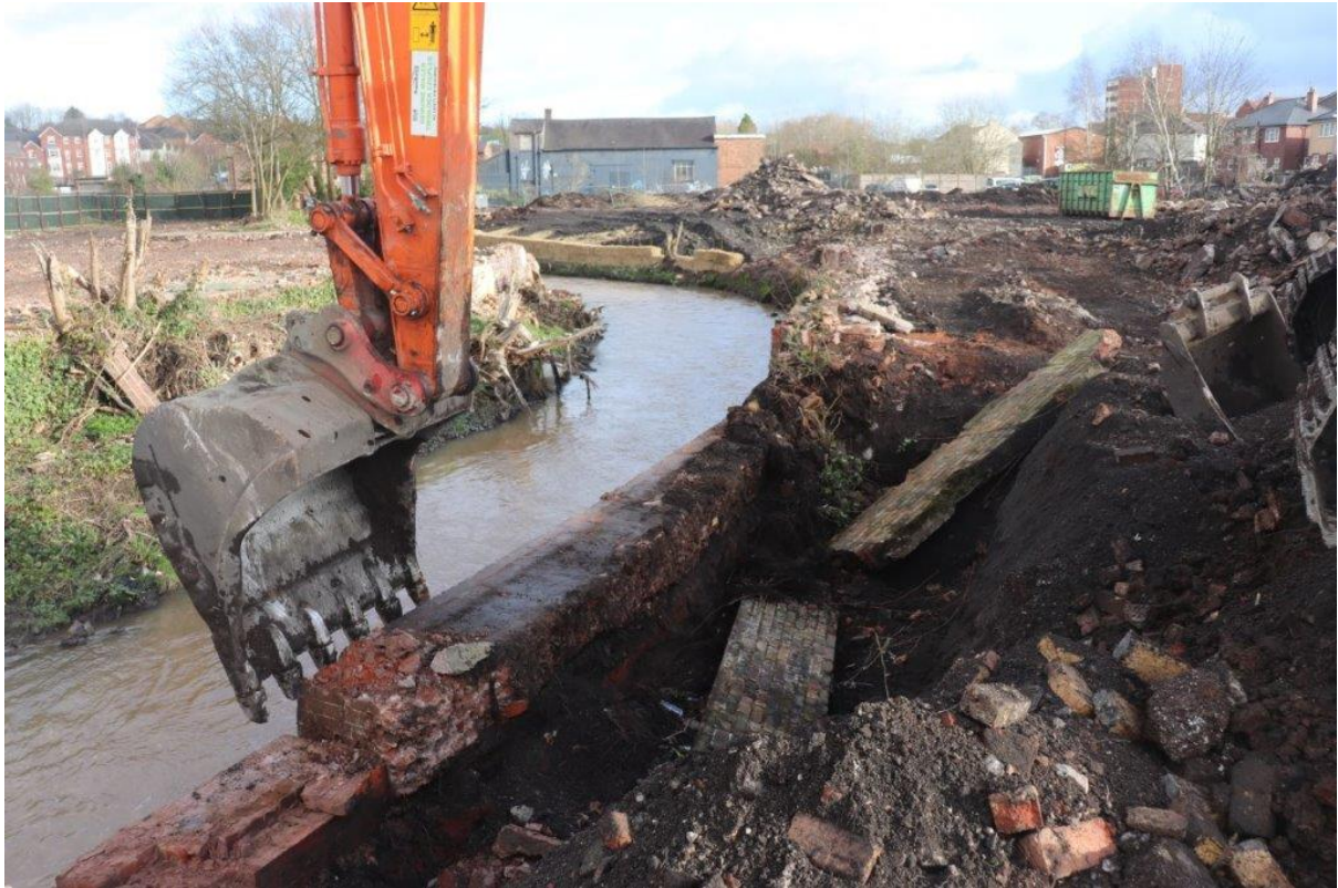
Plate 7: Collapsing retaining wall into trench, view east
