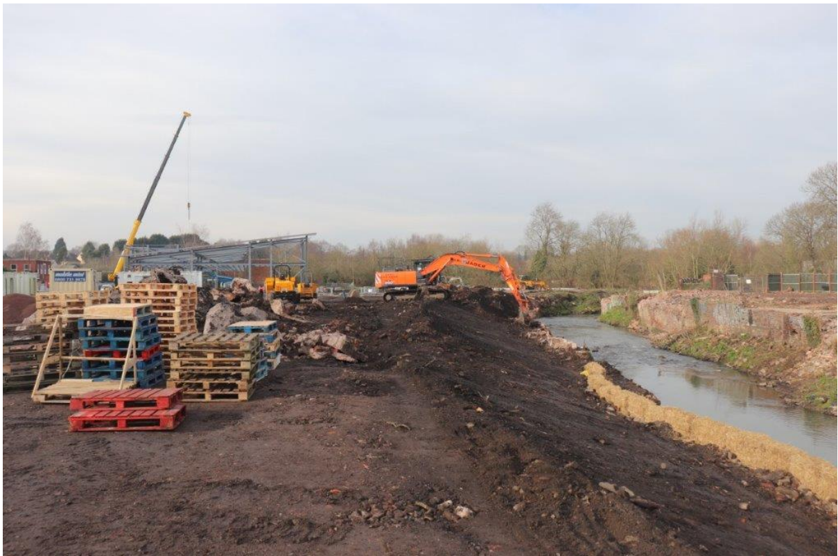
Plate 10: Profiling the western end of the site following removal of the retaining wall and modern foundations, view west
