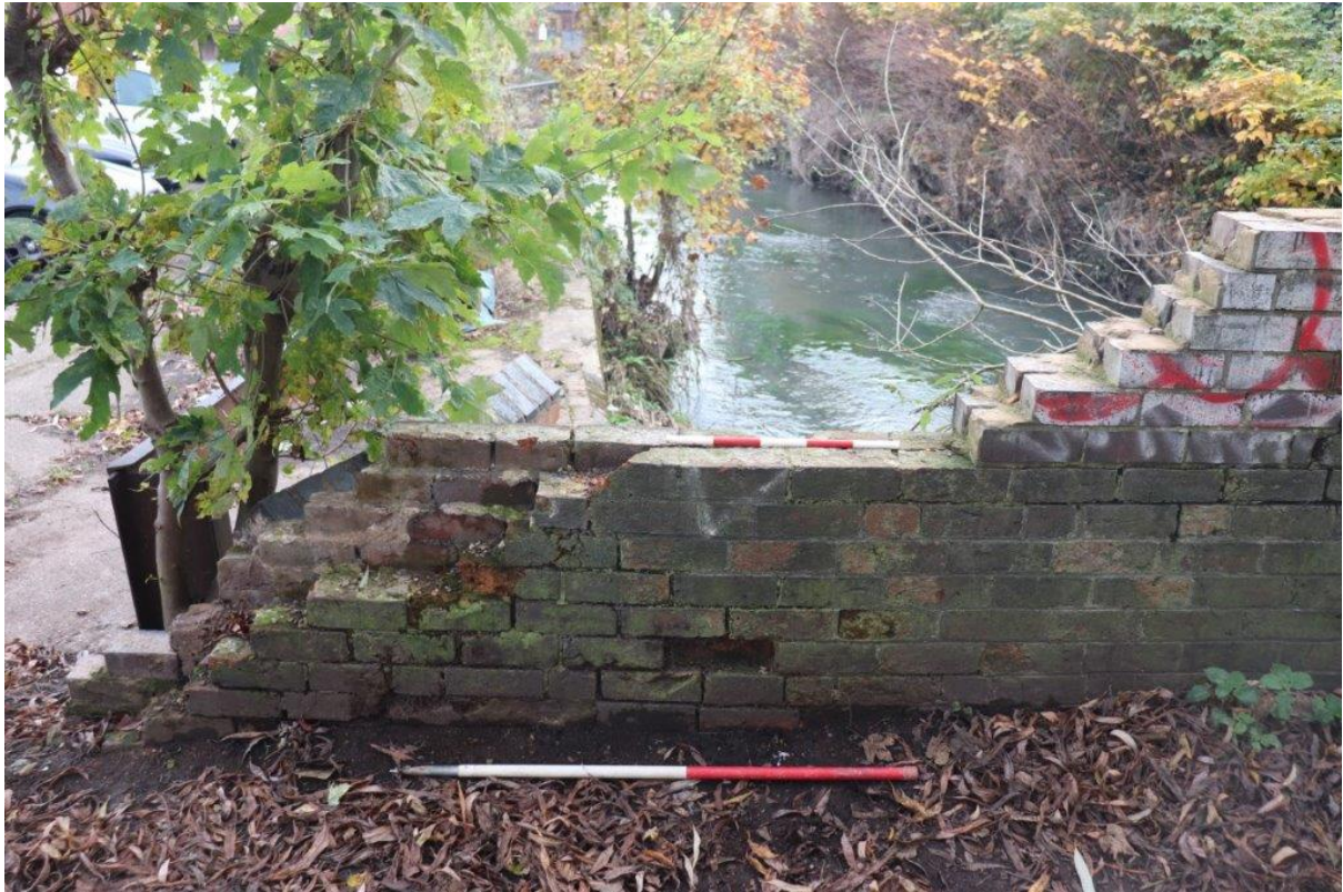
Plate 15: Brick wall at north-west side of bridge, view east , 0.5m and 1m scales
