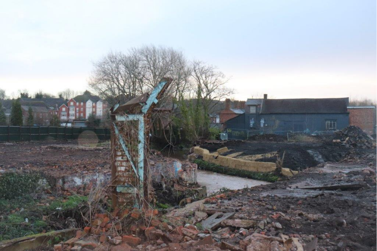
Plate 5: Remaining steel girder of existing building and general east view of the site
