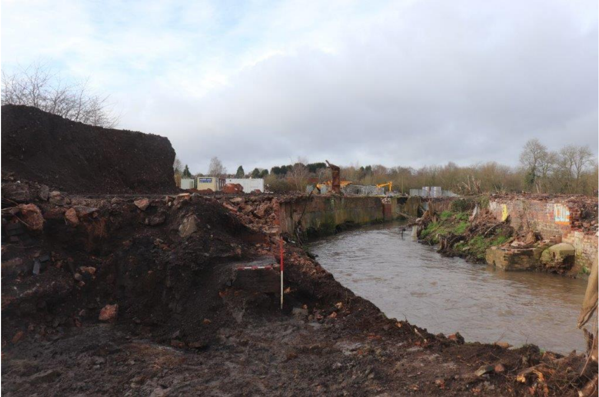
Plate 3: Retaining wall along the edge of the canalised river Stour, view west, 0.5m and 1m scales
