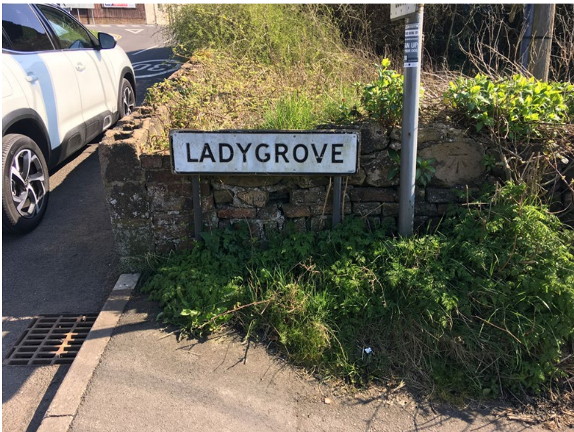
Plate 2 The wall, north end, at the junction of Ladygrove and Station Road, looking south-east
