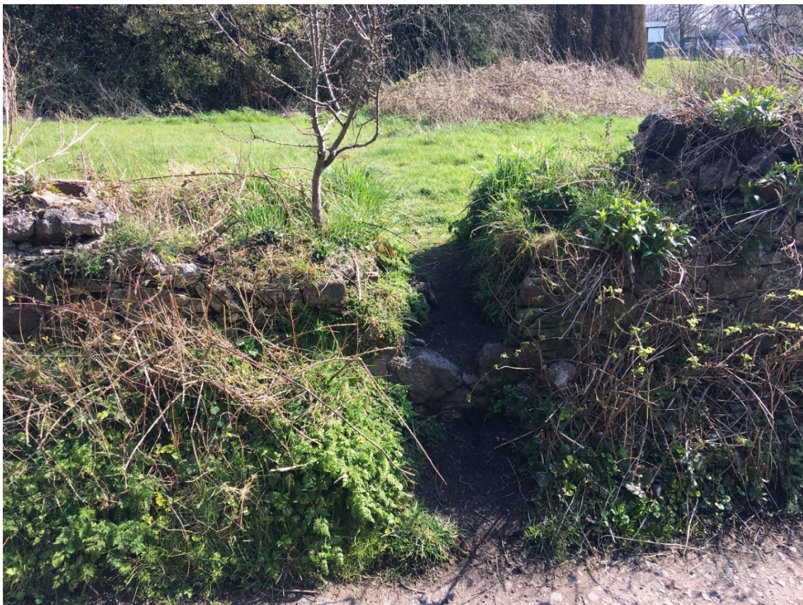
Plate 7 The wall showing some deterioration in its condition, looking south-east
