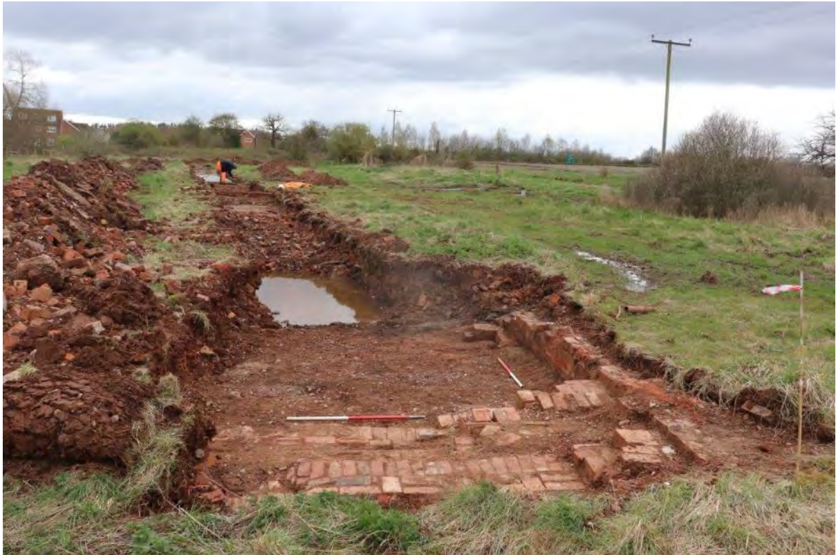
Plate 31: Looking south-west across Trench 92. Wall 9204 is visible in the foreground. 1m scales.
