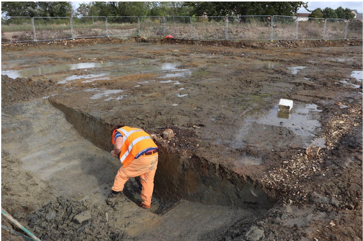
Plate 20: Excavating the large post-medieval orchard boundary ditch CG33 in the north of Parcel F.
