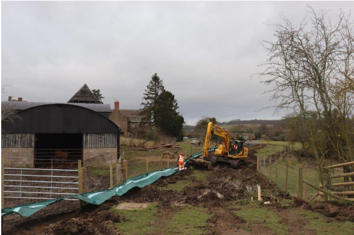
Plate 9: Location of trial hole for drain connection, during initial topsoil stripping in February. Looking north
