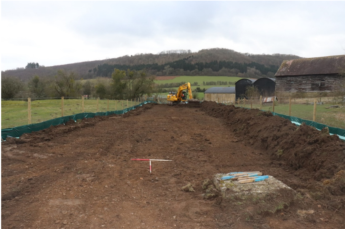
Plate 7: South end of Scheduled Monument area of Stokesay Castle following topsoil strip, with manhole in foreground. 1m scales looking south.
