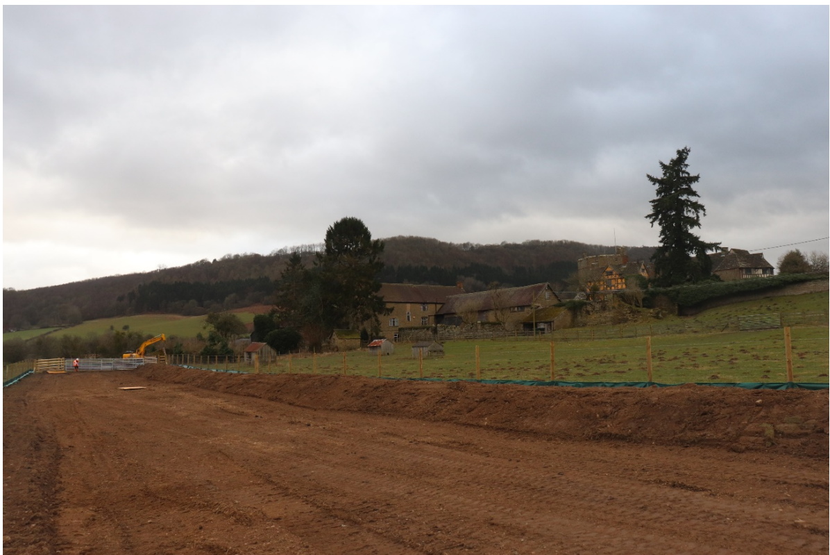
Plate 8: Easement topsoil strip with Stokesay Castle and StokeCastle farm in background, looking southwest.
