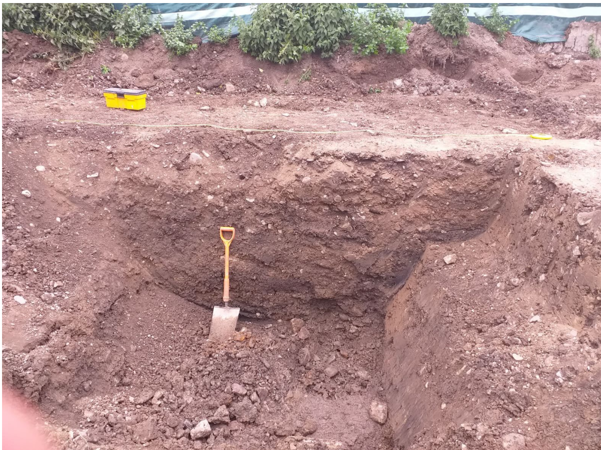
Plate 10: Trial hole for drain connection showing U-shaped drainage channel and backfill. Looking northwest, no scale.
