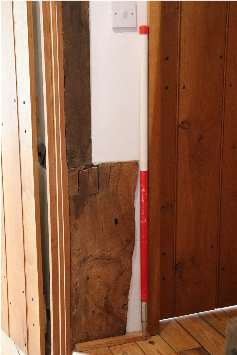
Plate 9 Phase 1 head of jowl post with tenon visible that would have jointed to the wall plate and tie beam, looking north-east, scale 1m
