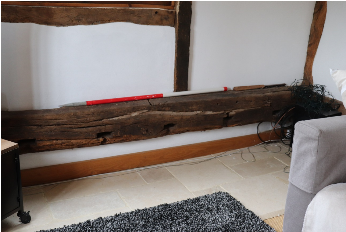
Plate 11 Re-used former floor joist within the Phase 2 additional southern bay, looking south, 1m scale
